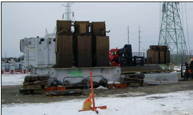
LEFT: Copper core bundles are visible in a power transformer that was removed by G&S from the X-533 Switchyard.
