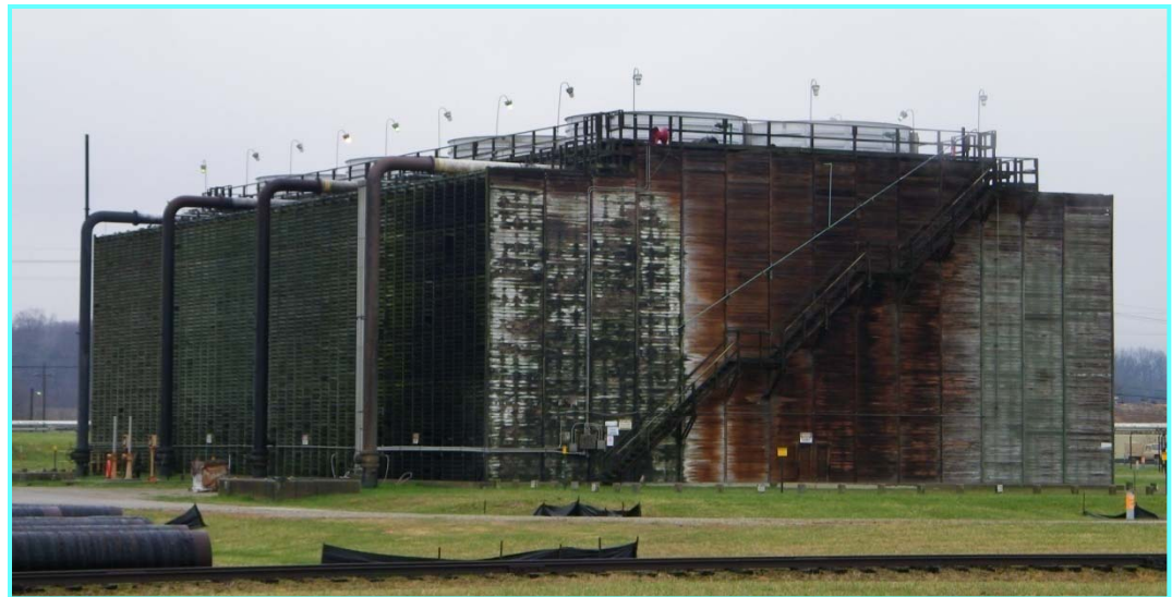
X-626 Recirculating Cooling Water Complex
