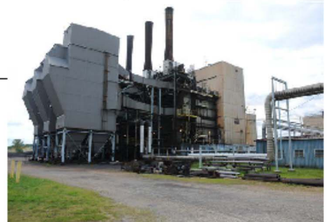
X-600 STEAM PLANT (OFF LINE ON 10/16/12)
