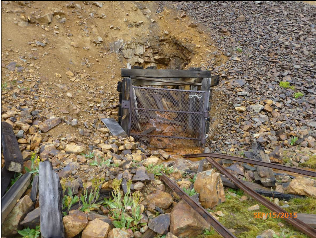
Figure 13. Photograph taken on September 15, 2015, showing acid seepage from the Blackhawk Mine located south of the Gold King Mine.
