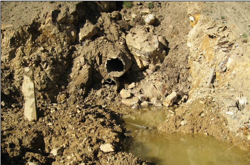
Figure 26.—Photograph showing the excavation of the Gold King Mine New Adit portal on September 11, 2014, taken shortly after the photograph in figure 23 (photograph from EPA project files).
