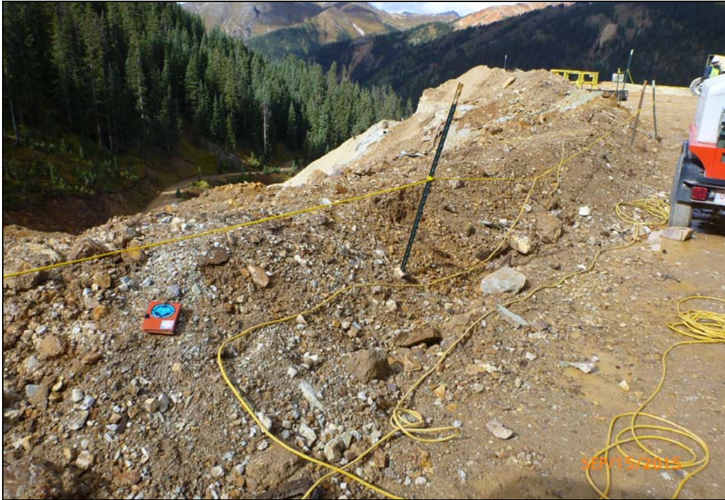
Figure C-1.—Photograph showing the safety berm made of soil that was excavated from in front of the Gold King Mine Level 7 New Adit portal. Sample No. 1 consisted of soil sampled from various locations along the safety berm.
