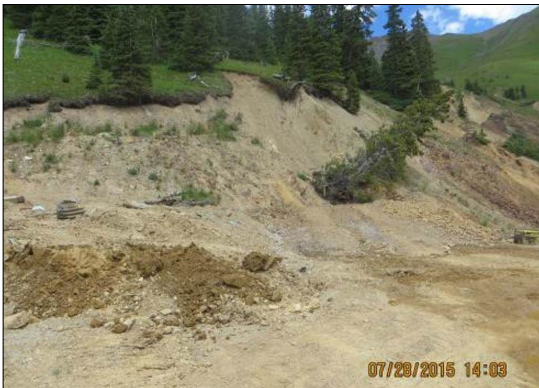
Figure 35.—Photograph showing the condition of the Gold King Mine Level 7 New Adit portal area on July 28, 2015. Note the soil and a tree that has slid downslope onto the portal area; at this time the seepage had been returned to the concrete trough, and the dump was drying out (photograph from EPA project files).
