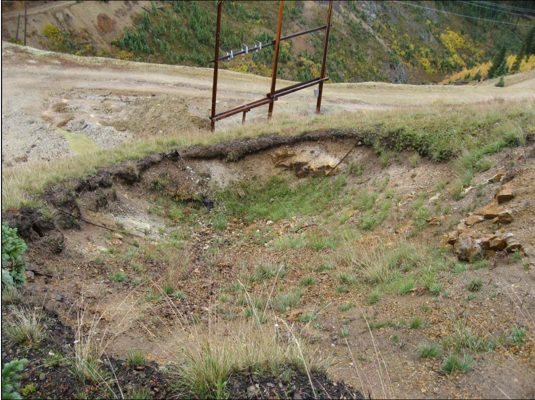
Figure 32.—Photograph taken on September 22, 2014, looking downhill at the subsidence pit located above the Gold King Mine Level 7 Old Adit.
