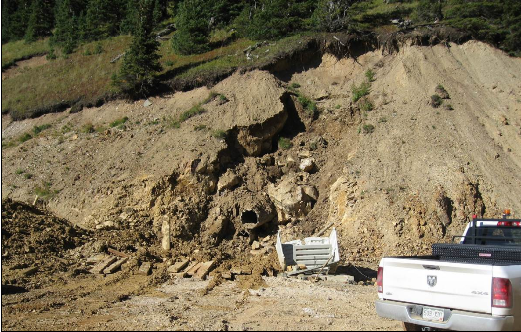
Figure 25.—Photograph showing excavation of the Gold King Mine New Adit portal on September 11, 2014. The metal grating and portions of the upper corrugated HDPE pipe and the lower solid-wall drain pipe have been removed (photograph from EPA project files).
