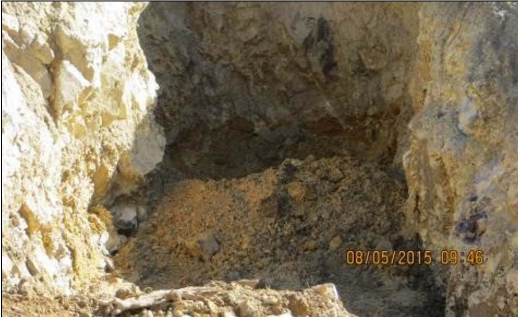
Figure 47.—Photograph taken at 9:46 a.m. August 5, 2015, showing that the loose soil from the upper end of the excavation had been removed exposing fractured and crumbly rock (photograph from EPA project files). The fill derived from the excavation had now covered the timbers, lagging, and seep visible in the previous photograph (figure 46). This indicates that the bottom of the excavation was about 10 feet above the level of the floor of the adit; this corroborates reports that they were digging high, trying to stay above the assumed water level in the adit.
