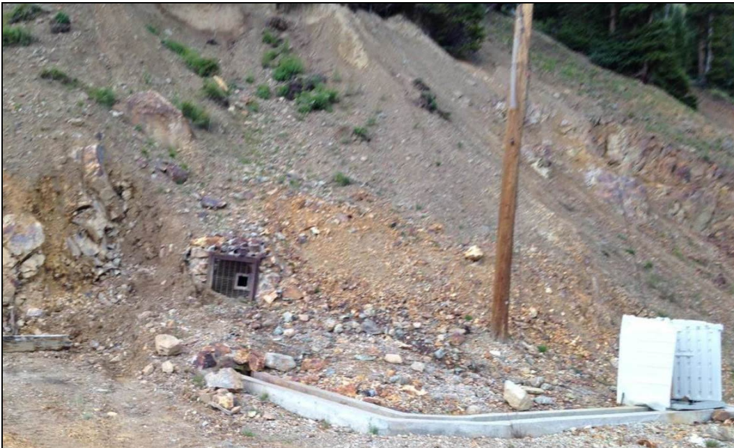
Figure 22.—Photograph showing the condition of the Gold King Level 7 New Adit portal on August 27, 2014, prior to any EPA modifications. Soil and rock debris have migrated downslope and covered a portion of the drain installed in 2009 (photograph from EPA project files).
