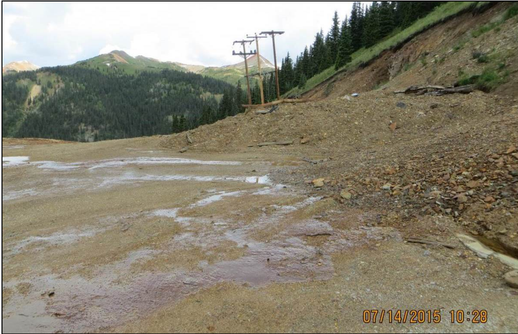
Figure 33.—Photograph showing the condition of the Gold King Mine Level 7 Old Adit portal area on July 14, 2015. Note that more soil and rock had slid from the slope area and had buried a portion of the concrete diversion channel including the ends of the two drain pipes (photograph from EPA project files).
