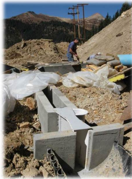
Gold King Level 7 Old Portal with 2" Parshall Flume Installed in Concrete Lined Ditch
