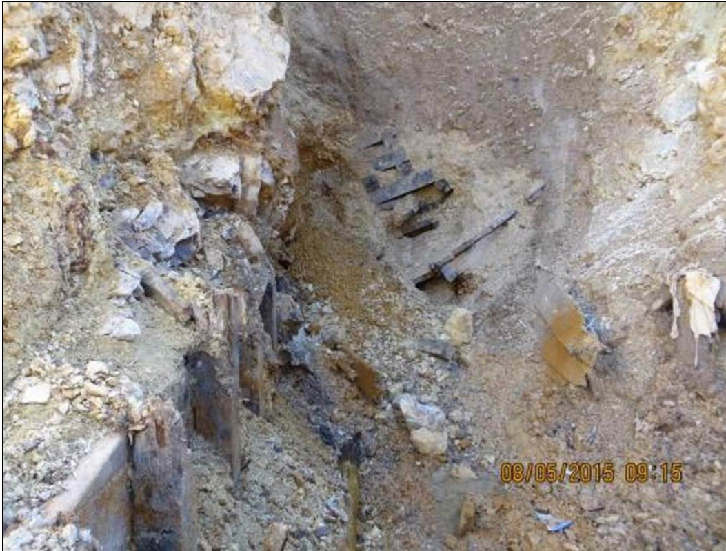
Figure 46.—Photograph taken at 9:15 a.m. August 5, 2015, showing the Gold King Mine Level 7 New Adit excavation uncovering mine timbers and lagging (photograph from EPA project files). Minor seepage is visible just to the left of the date stamp where a small puddle has formed. Note the soil in the upper end of the excavation above the timber lagging.
