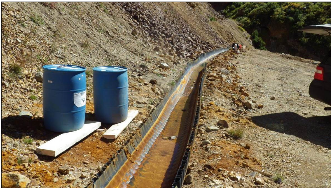
Figure 24.—Photograph showing seepage flow in the half-pipe channel at the Gold King Mine Level 7 New Adit area on September 11, 2014. Flow of approximately 12.6 gpm was recorded (photograph from EPA project files).
