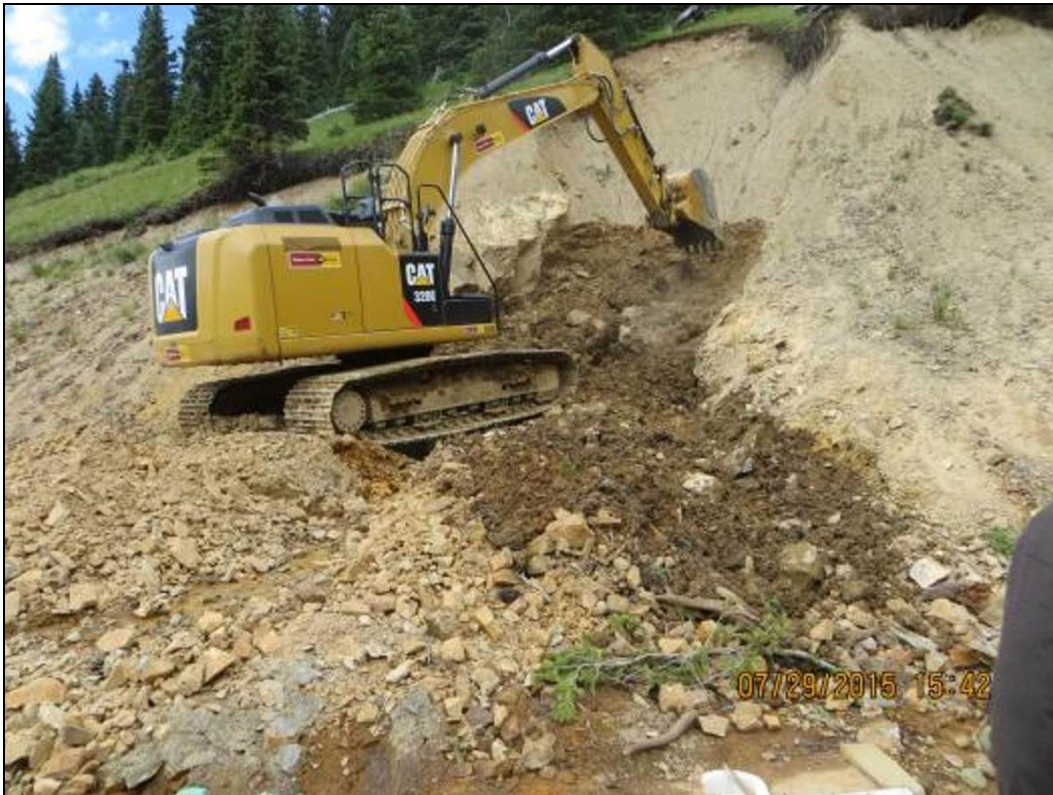
Figure 36.—Photograph taken on July 29, 2015, showing initial excavation work at the Gold King Mine Level 7 New Adit that was performed to remove the additional accumulation of debris from the eroding slope above the adit (photograph from EPA project files).
