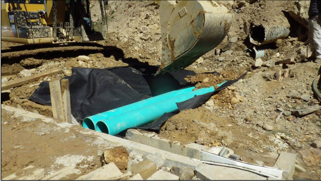
Figure 28.—Photograph taken on September 11, 2014, showing the installation of two new 2-foot-diameter drainage pipes. An entrance slot has been cut into the concrete trough for the pipes to discharge into (photograph from EPA project files).
