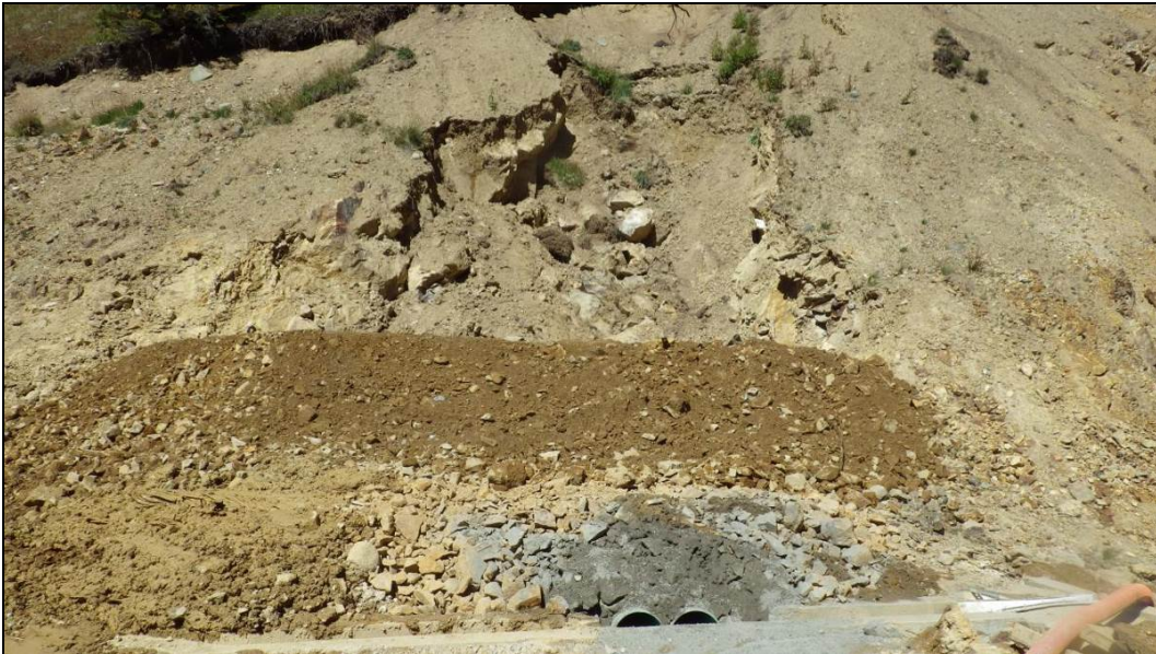
Figure 29.—Gold King Mine Level 7 New Adit as it appeared on September 12, 2014, when EPA completed placing backfill over the two new drain pipes. Note that a steep slope was left in place in the mountainside above the drain pipe installation (photograph from EPA project files).
