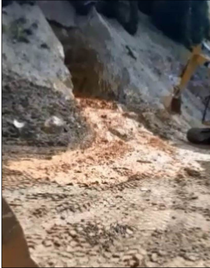
Figure 52.—Photograph showing the initial blowout from the adit. At this point, the flow is surging up over the backfill that was present in the portal area (still frame extracted from a video taken on August 5, 2015, at approximately 10:55 a.m.).
