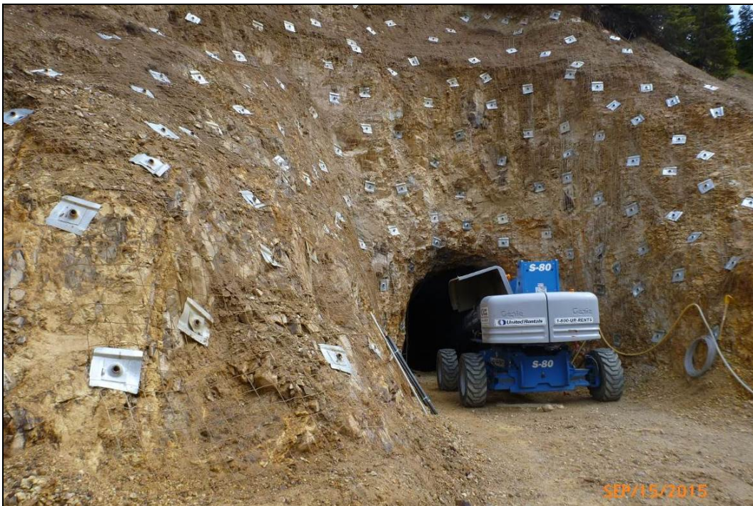
Figure 65.—Photograph taken on September 15, 2015, showing the installation of wire mesh and rock bolts to stabilize the outside of the mine opening.
