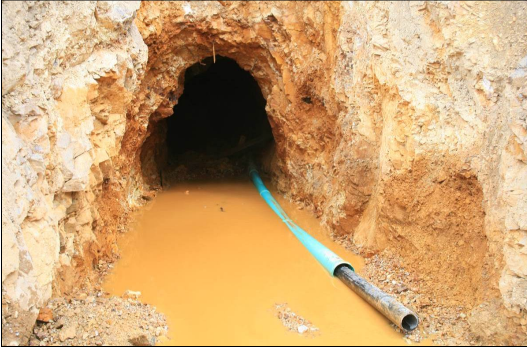
Figure 63.—Photograph showing the adit on August 16, 2015, with an 80-ft long (four 20-foot segments) turquoise-colored 24-inch outside-diameter drain pipe inserted into the adit opening. An 8-inch inside-diameter black HDPE pipe has been inserted into the 24-inch diameter pipe.
