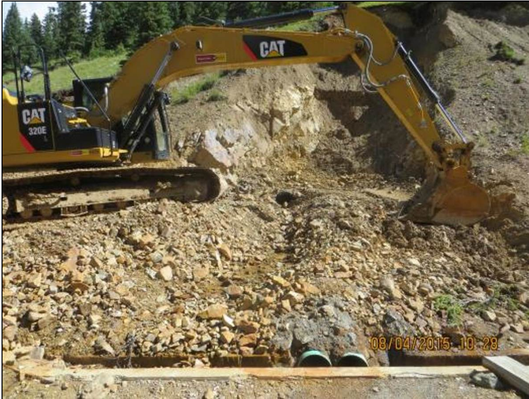
Figure 37.—Photograph showing additional excavation at the Gold King Mine Level 7 New Adit at 10:28 a.m. August 4, 2015 (photograph from EPA project files).
