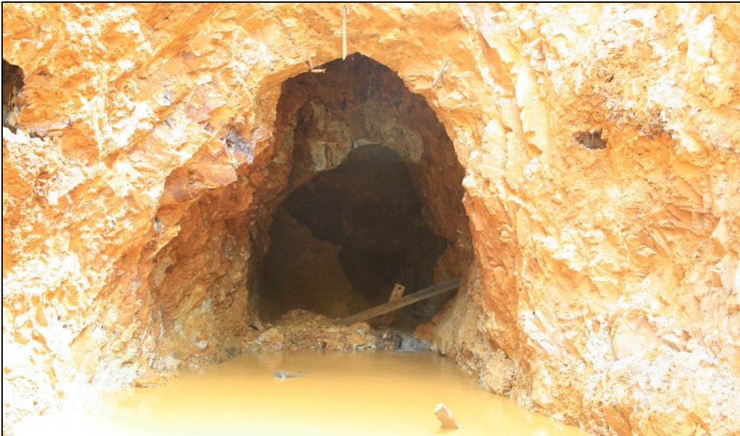
Figure 62.—Photograph showing the Gold King Mine Level 7 New Adit on August 16, 2015, after an excavator was used to reach inside the mine opening and remove the timbers. Note piles of debris from partial roof collapses inside the adit.
