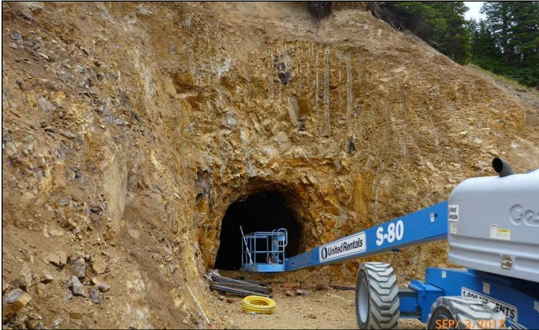
Figure 64.—Photograph showing the adit on September 3, 2015, at the initiation of rock bolting. The rock had been excavated to provide a larger work area. Note the excavator teeth marks left in the rock, an indication that the rock is altered and contains a significant amount of clay.
