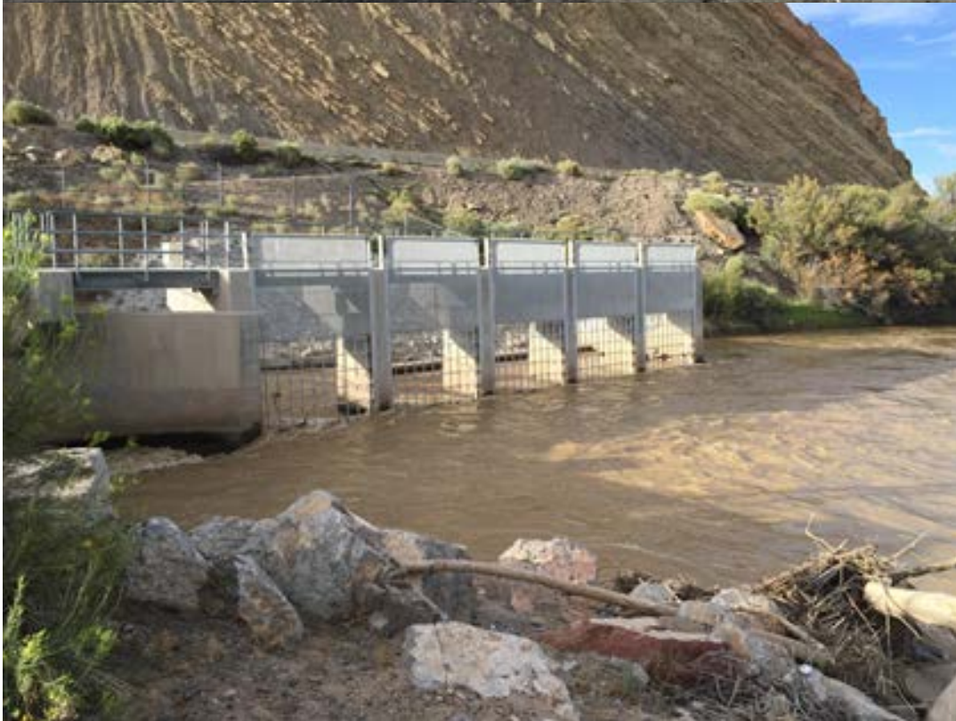
Figure 6. Sampling location for samples collected by BOR at the Hogback Diversion Channel.
