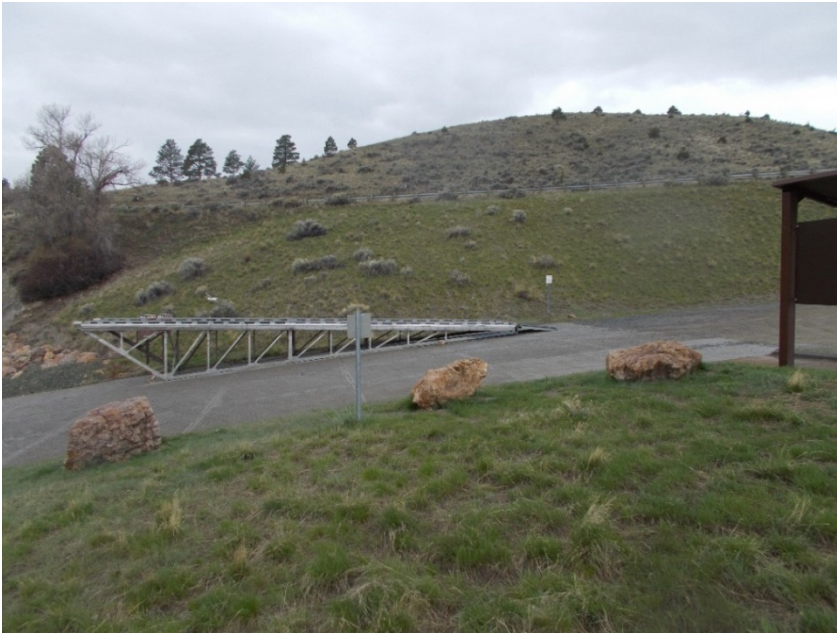
Figure 5: Shannon Recreation Area Courtesy Boat Dock. Image is taken after the incident. Access Ramp is in an open position in contact with the ground. Image courtesy of the Lewis and Clark County Sheriff's Department.
