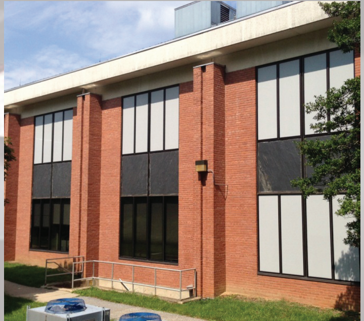
White Standard CollidEscape window film on East Façade and South Façade Windows of the USGS Gabrielson Laboratory at Patuxent Research Refuge, Maryland. Photo credit: US Fish and Wildlife Service
