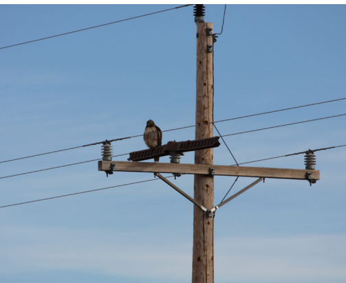
A device to protect raptors from electrocution installed on new utility poles at DOE's Pantex Plant. Photo: DOE
