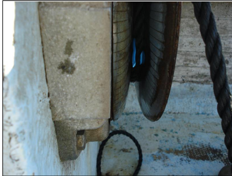
Figure 2-4 Tag Fouling in the Winch Pulley
