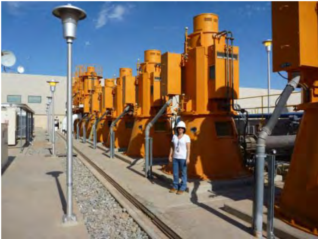
Photograph 4. High-pressure reverse osmosis pumps.
