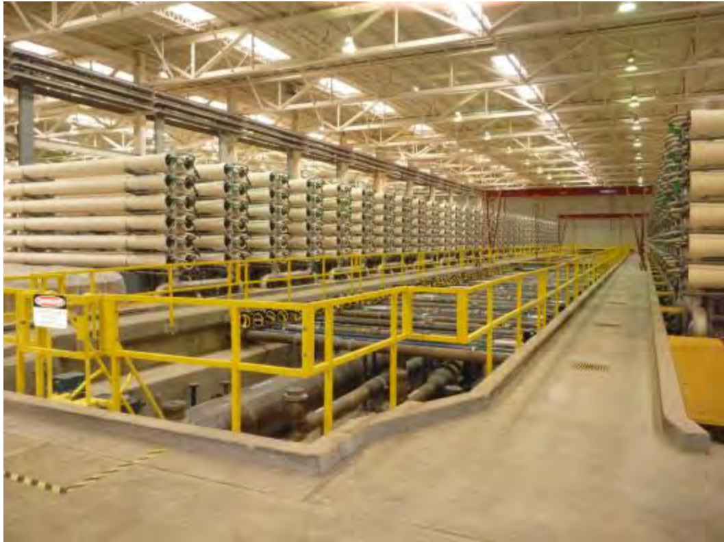
Photograph 2. Fluid Systems reverse osmosis area.
