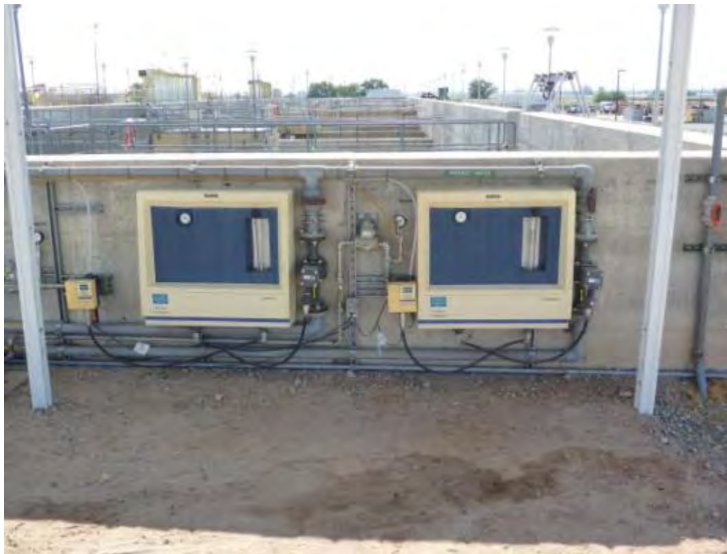
Photograph 5. Instrumentation associated with the temporary ammonia system.
