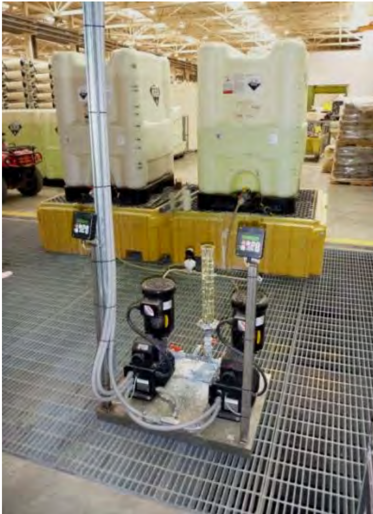
Photograph 6. Chloramines neutralization equipment.
