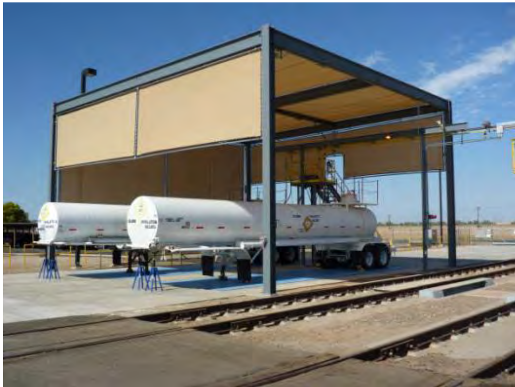
Photograph 3. Chlorine tanker facility.
