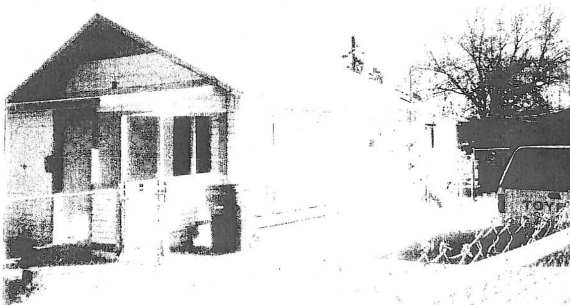
Porch and south façade of residence at 165 W. Fifth Ave. Note boarded-up window with air-conditioner, rolled asphalt roof, and rear addition.
