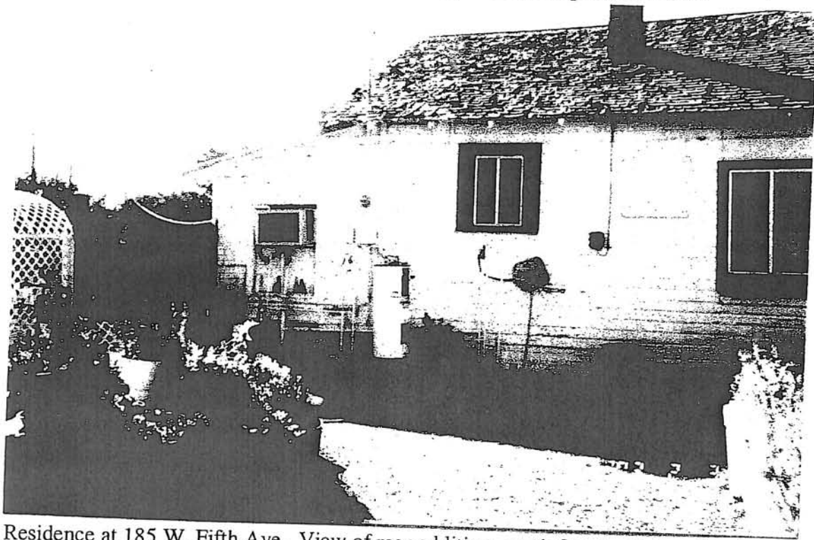
Residence at 185 W. Fifth Ave. View of north façade and front porch. Note boarded-up window holding air conditioner and wood shingles on north portion of roof.
