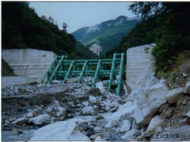
Photo 16. Open grid-type check dam Source: Mizuyama, T (2008) Structural Countermeasures for Debris Flow Disasters
