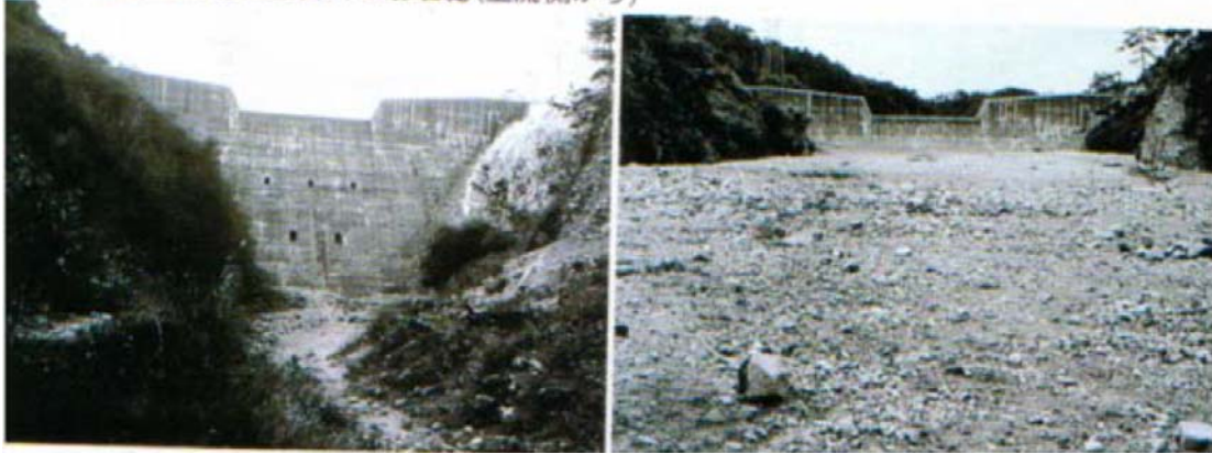
Photo 14. Closed-type concrete check dam in Sumiyoshi River, Rokko Mountain, Japan, 1967. Source: Mizuyama, T (2008) Structural Countermeasures for Debris Flow Disasters
