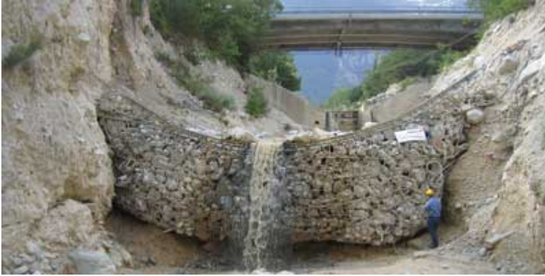
Photo 12. A flexible ring-net barrier that is impounding debris. Notice the sediment laden water that is passing through the structure. Source: http://www.geobrugg.com
