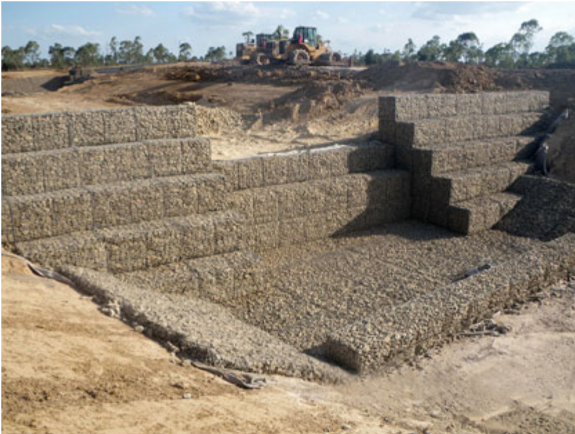
Photo 17. Gabion check dam in Moranbah, Queensland, Australia. Notice the Reno-mattress placed downstream of the check structure for scour protection. Photo by Prospect Contractors, Australia. http://www.prospectcontractors.com.au/anglo_coal.html
