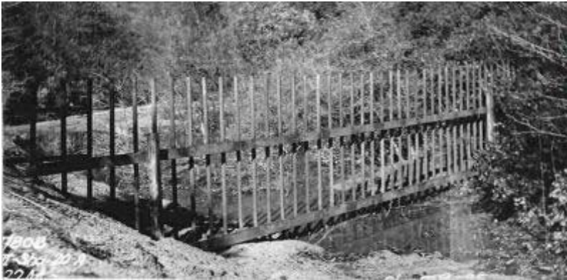
Photo 11. A debris rack/fence (no fence fabric) used to capture material upstream of a culvert. Photo courtesy of the Federal Highway Administration.
