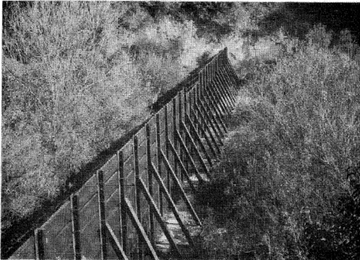
Photo 13: Debris Barrier Wall in Southern California. Source: USACE (1993) Assessment of Structural Flood-Control Measures on Alluvial Fans
