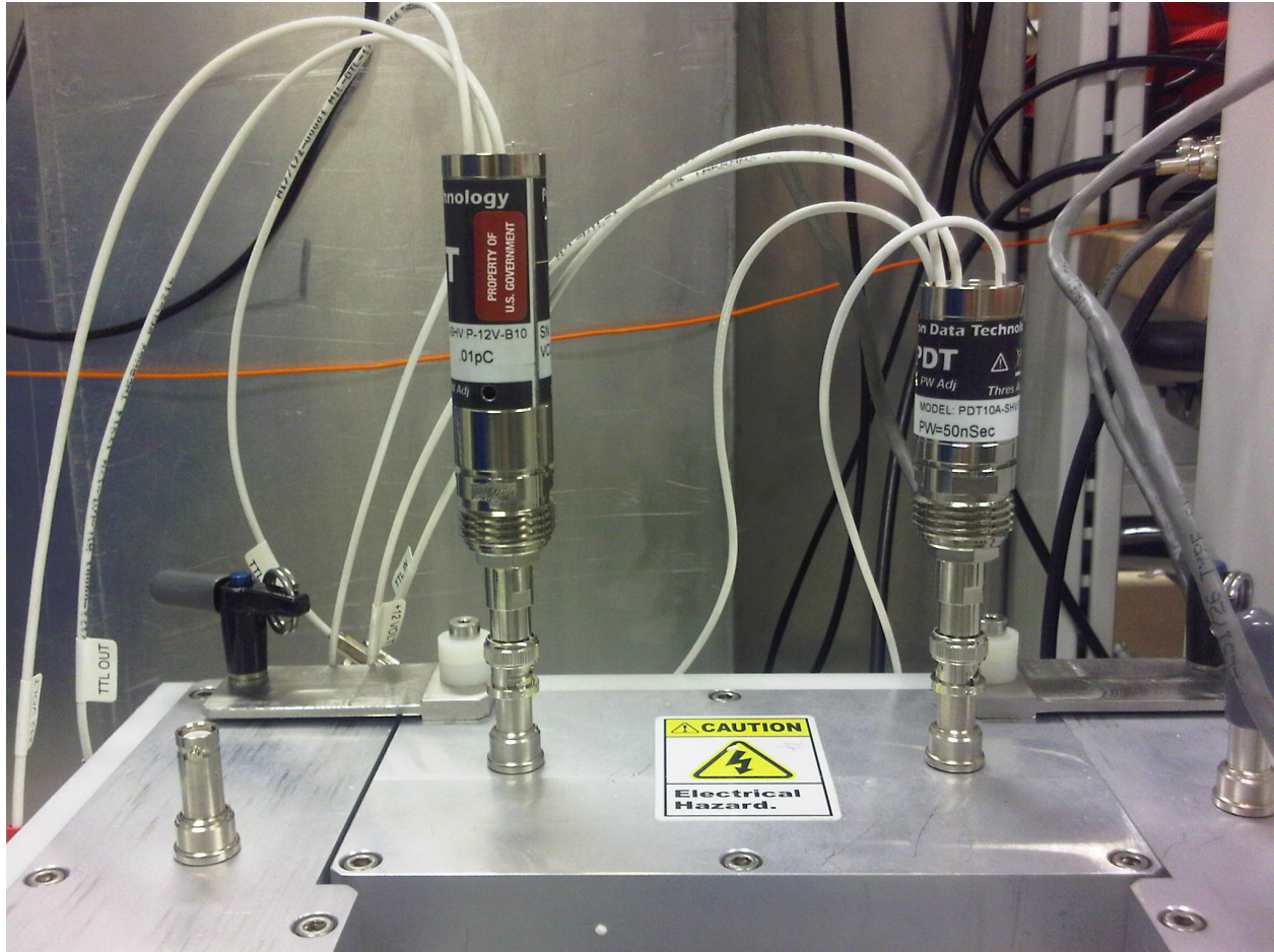
Figure 3.7. Preamps in place on one module.
