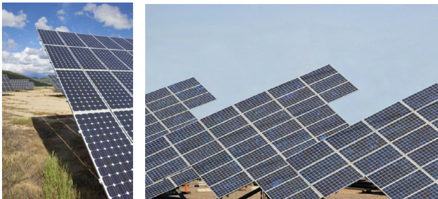
FIGURE 13.2 SIERRA SUNTOWER PV TECHNOLOGY
