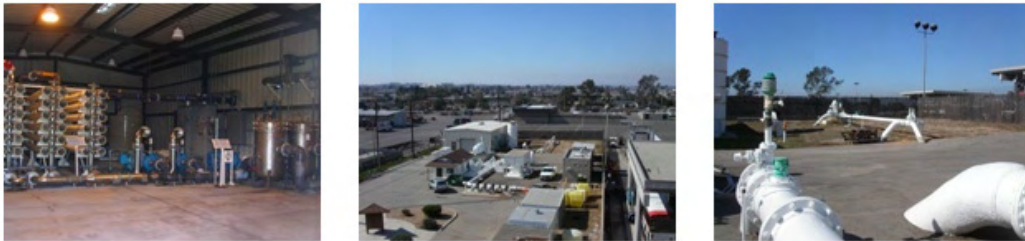
FIGURE 7.1 C. MARVIN BREWER GROUNDWATER DESALTER
