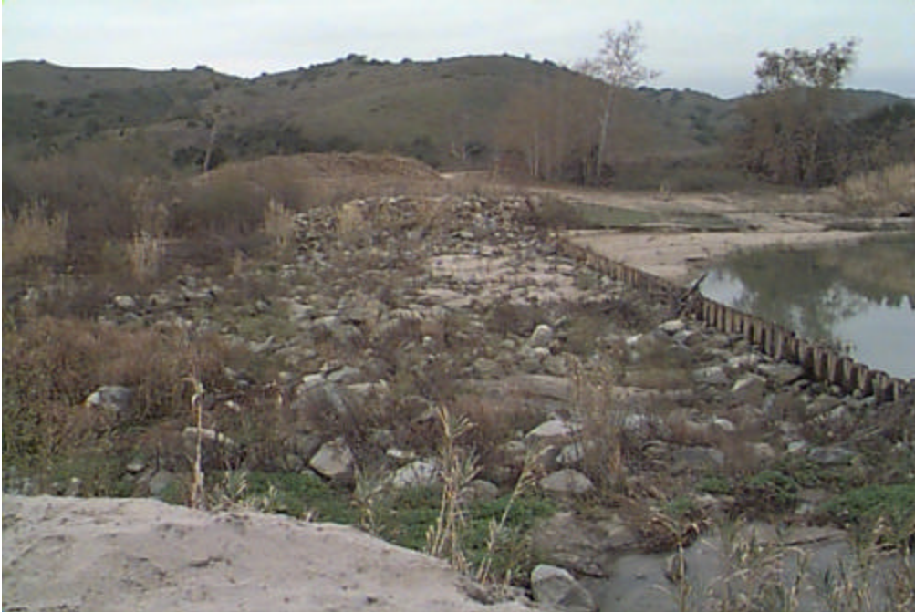
Figure 3. Looking from east bank across diversion weir after dredging of upstream reservoir was accomplished to reduce sedimentation. Dredge piles were placed on both sides of the river. Several rocks were estimated to have been placed at the toe of the dam after the 1993 flood. These rocks have since been washed a small distance downstream during subsequent floods as observed in this photo (2-8-99). Photo provided by West Consultants.
