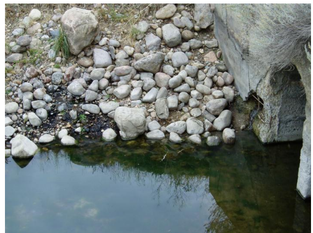
Figure 1.4 – Seepage around North Canal Outlet
