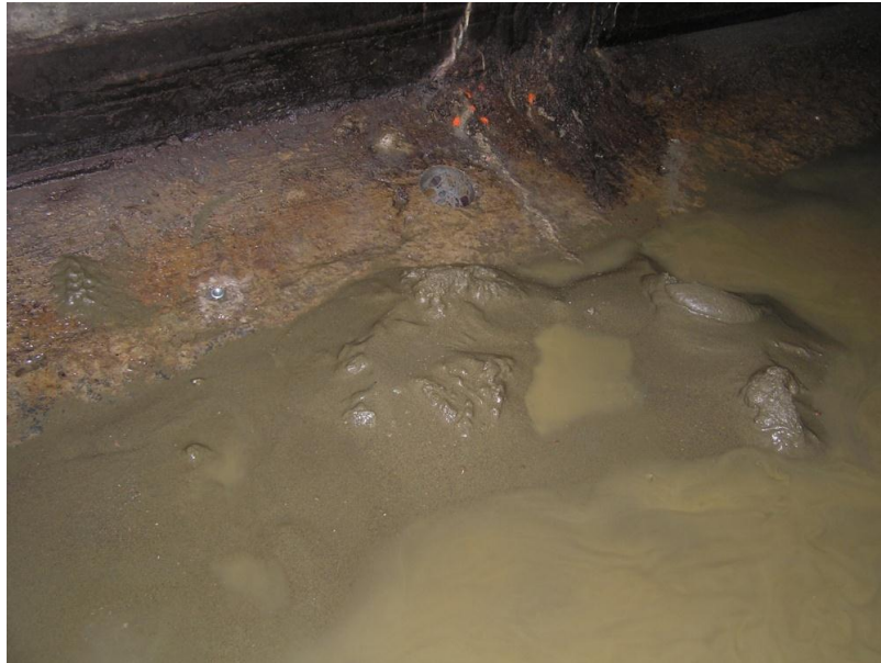
Figure 1.2 – Embankment Piping into Outlet Works Conduit
