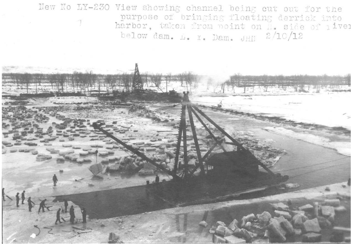
Figure A4. Clearing ice from the river to repair the apron Feb. 1912.
