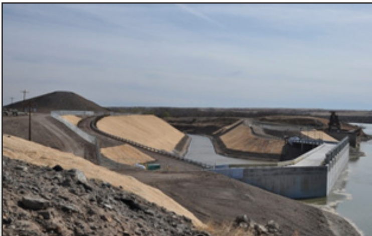
New headworks and fish screens at Intake Dam with screens submerged
