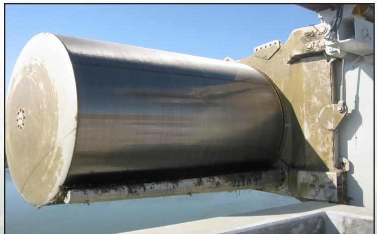
Close-up view of rotating drum and fish screen
