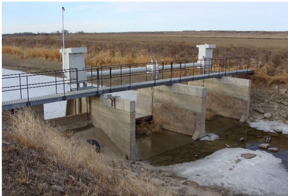
Figure 2-16. Example Check Structure
