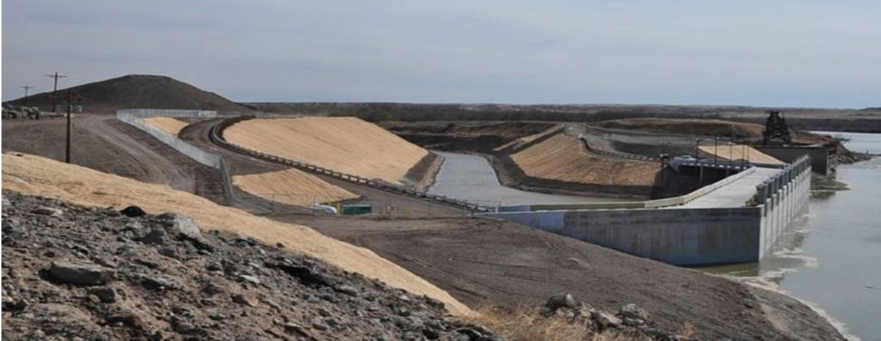
Figure 3-26. New Headworks at the Entrance of the Main Canal with Fish Screens Completed in 2011
