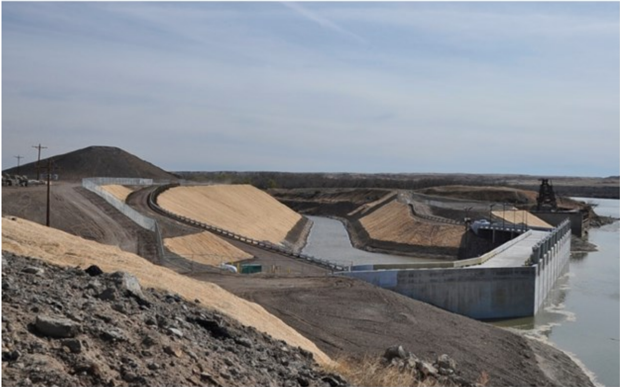
Figure 1-4. New Headworks and Submerged Fish Screens at Intake Diversion Dam
