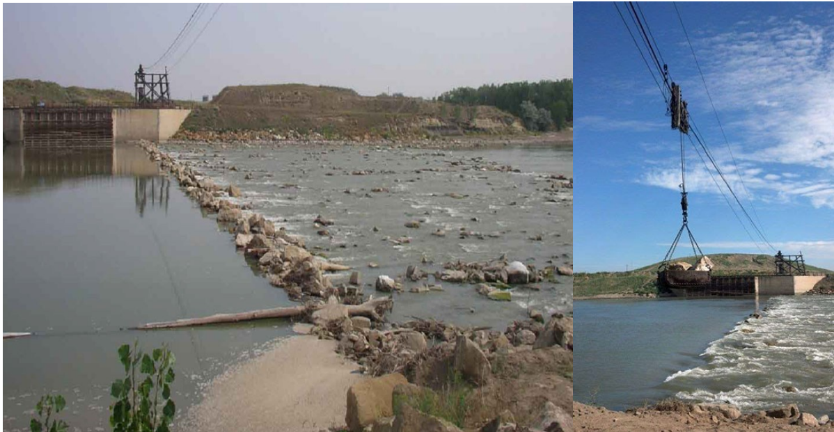
Figure 3-25. (Left) Low Water Exposes the Intake Diversion Dam Rock Weir; (Right) Higher Waters Create Riffle, Overhead Cableway Delivers Rocks to Weir
