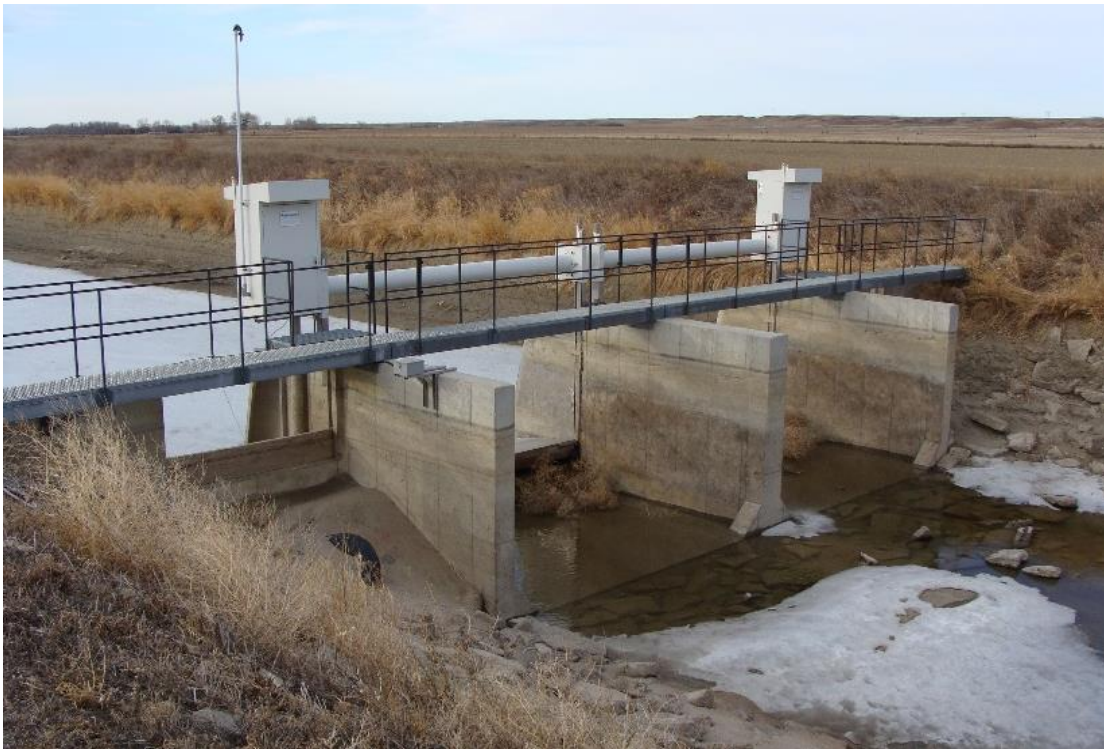
Figure 2-16. Example Check Structure
