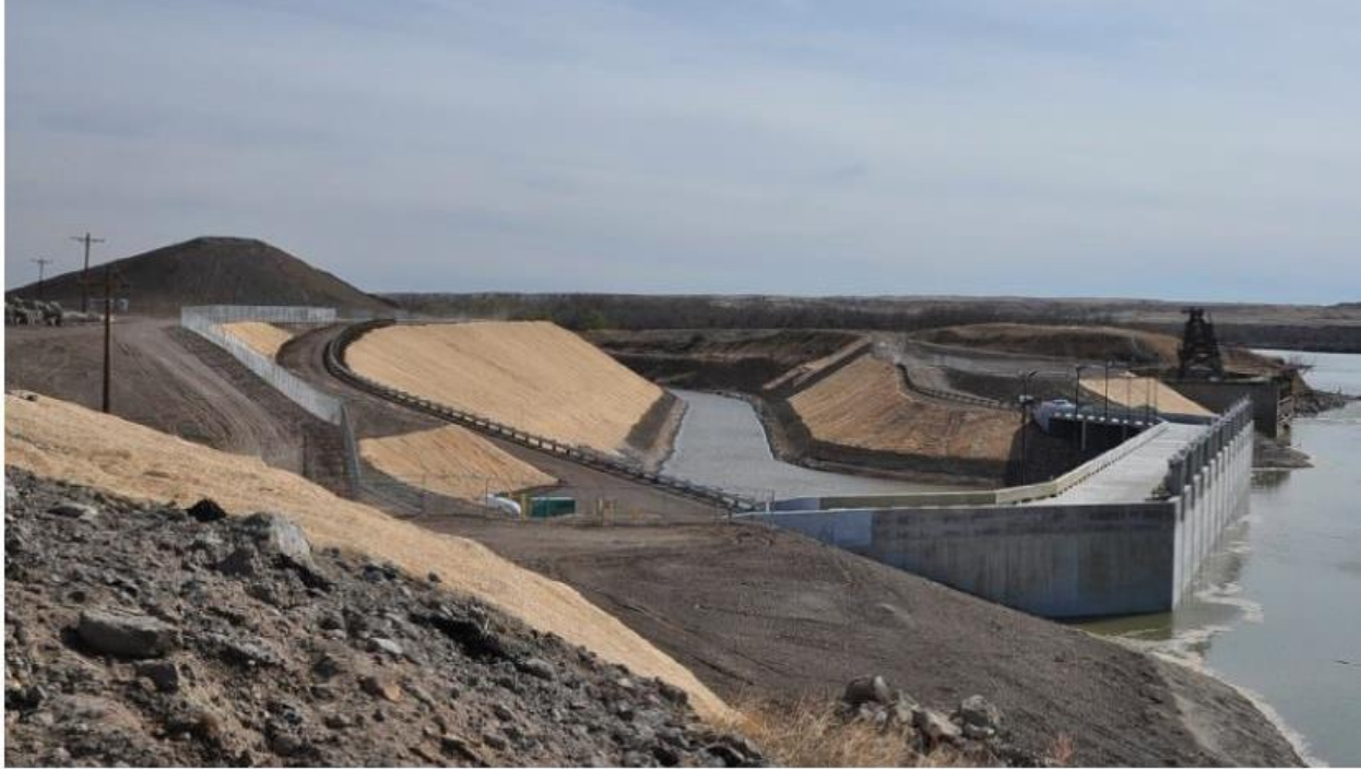
Figure 2-1. New Headworks and Fish Screens at Intake Diversion Dam
