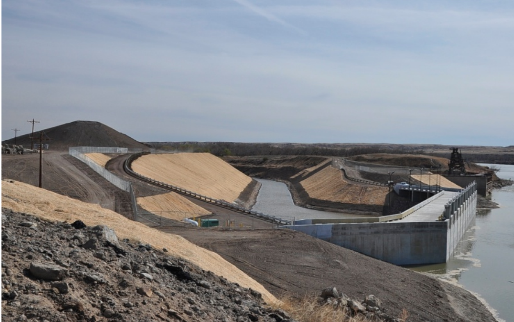
Figure 2-1. New headworks and fish screens at Intake Dam with screens submerged
