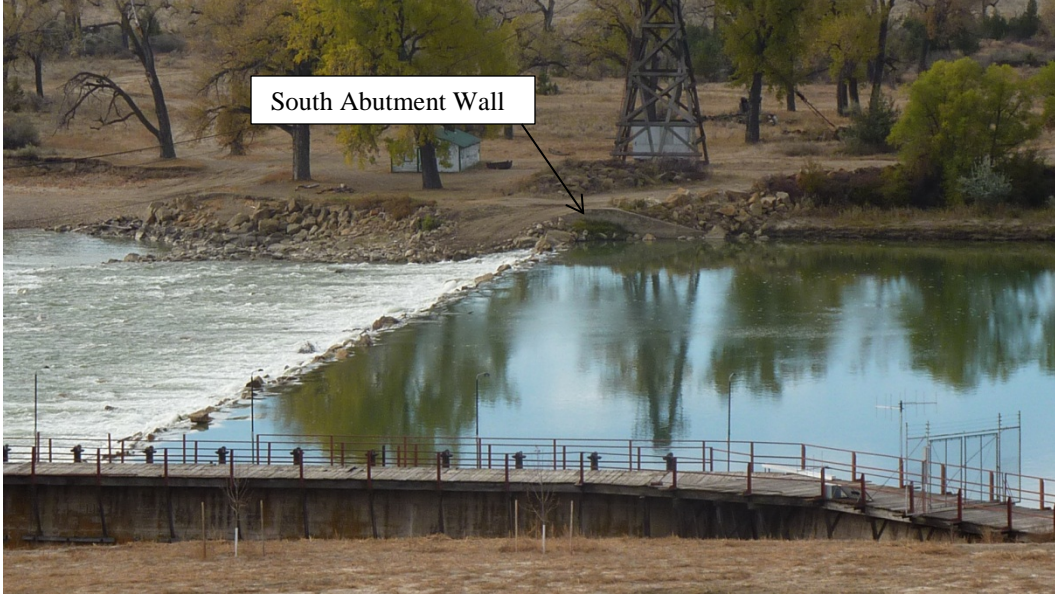
Figure 12. Existing dam showing old headworks structure (foreground) and south abutment concrete wall.
