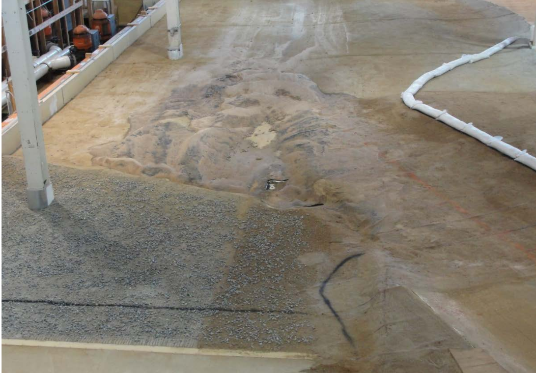
Figure 22. Sand scour after preliminary erosion test. It is likely that the existing scour hole will continue to scour in the future.
