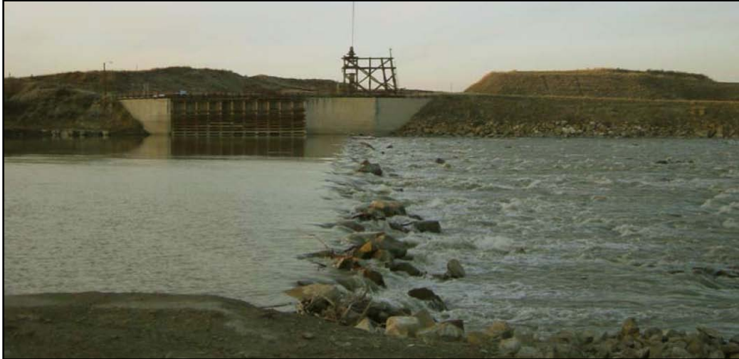
Figure 2. Lower Yellowstone Diversion Dam today with large rock dumped along the dam crest that has migrated downstream over the years preventing fish passage.
