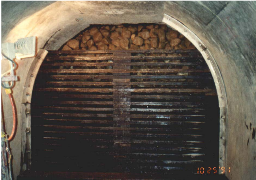
Figure 5. Photograph taken on October 25, 1991 of the Timber-Lattice Bulkhead as construction was nearing completion showing the layer of cobbles at Station 4+62 of the LMDT.
