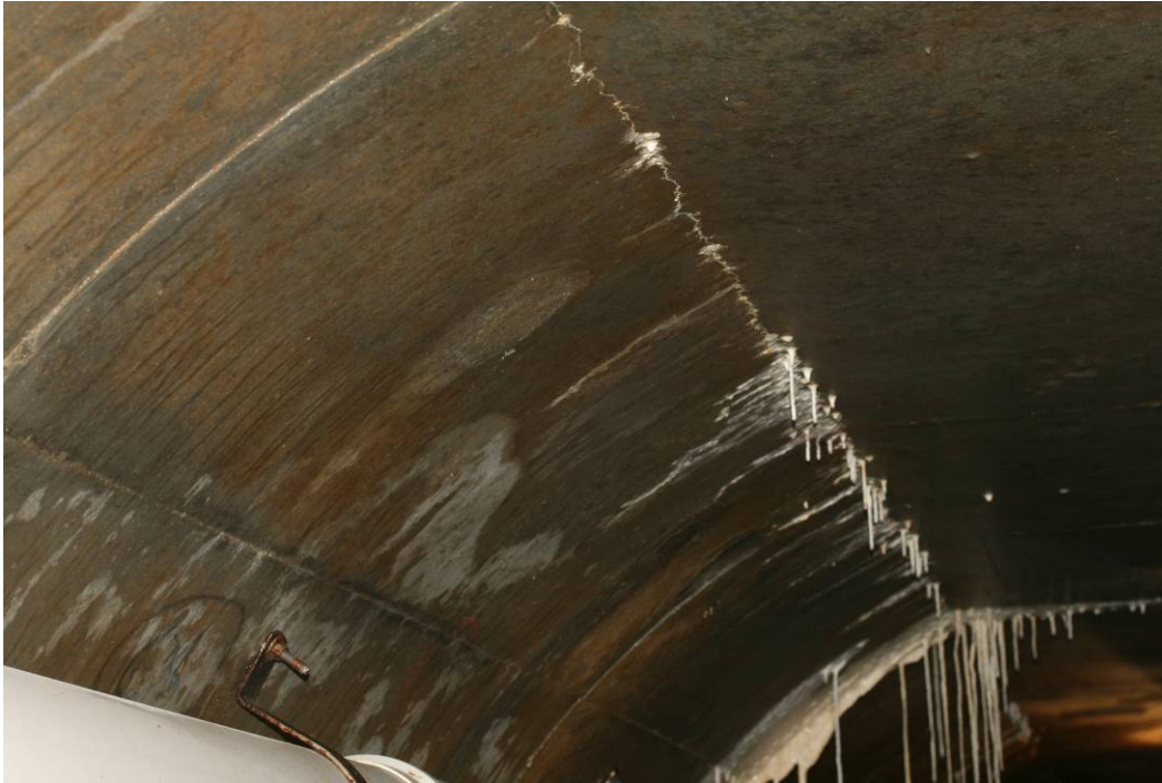
Figure 20. Photograph taken on March 25, 2008 looking downstream from about midway inside the reinforced concrete lined segment of the LMDT. Note the calcium carbonate stalactites forming from the slow seepage along a thin roof crack and at a joint in the concrete lining.
