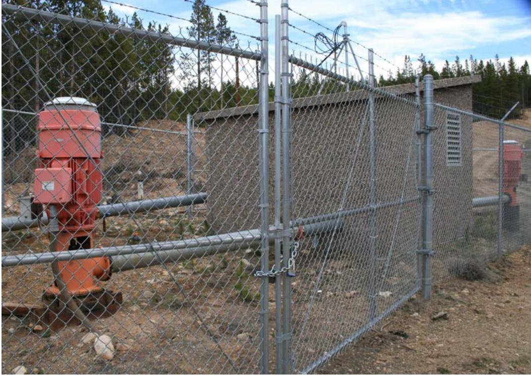
Figure 29. View of Pumphouse and Extraction Wells in the vicinity of Station 10+25. May 28, 2008.
