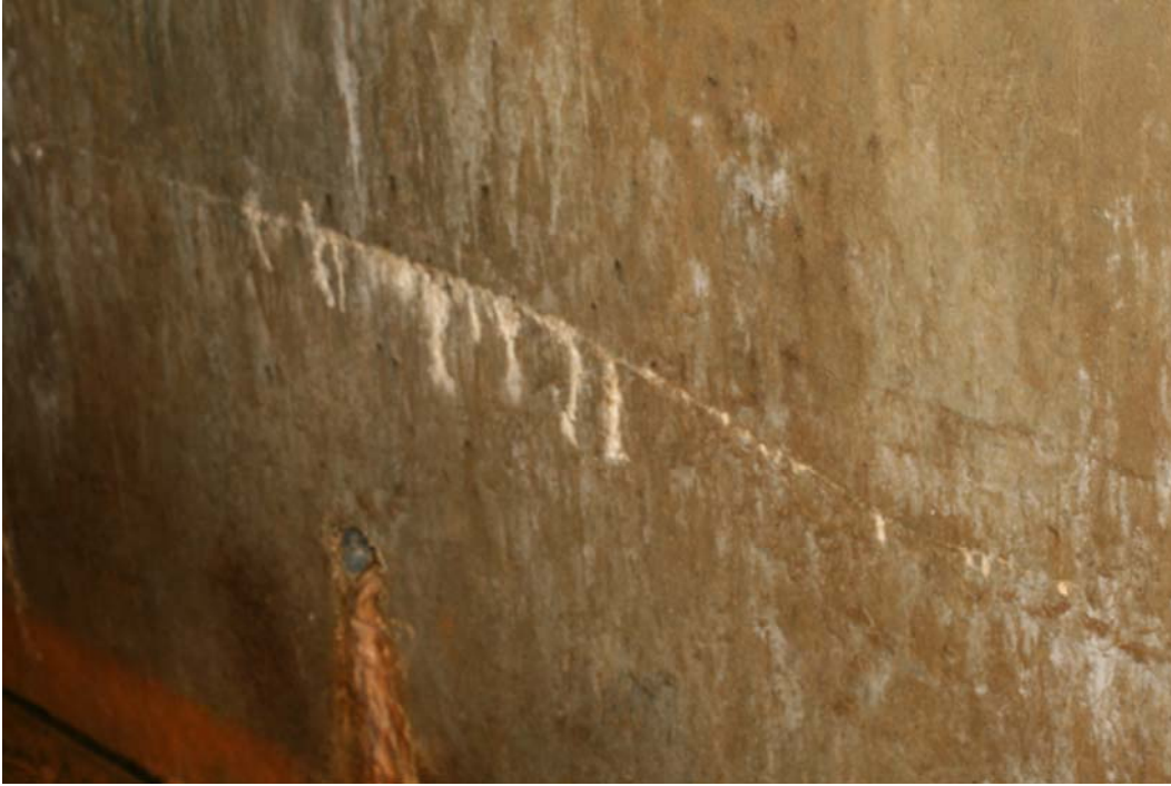
Figure 21. This crack located about 3 feet above the LMDT floor is the only one that showed offsetting of the concrete. The offset is about 1/8 inch.
