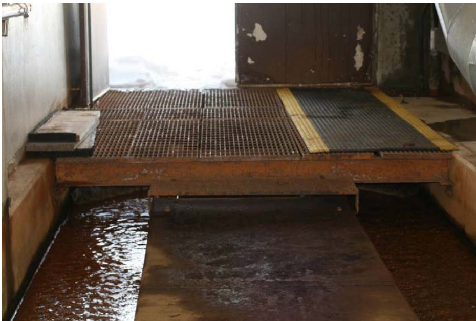
Figure 18. Photograph taken on March 25, 2008 looking at the downstream end of the LMDT showing the concrete center walkway with drainage ditches on either side and steel floor grating.
