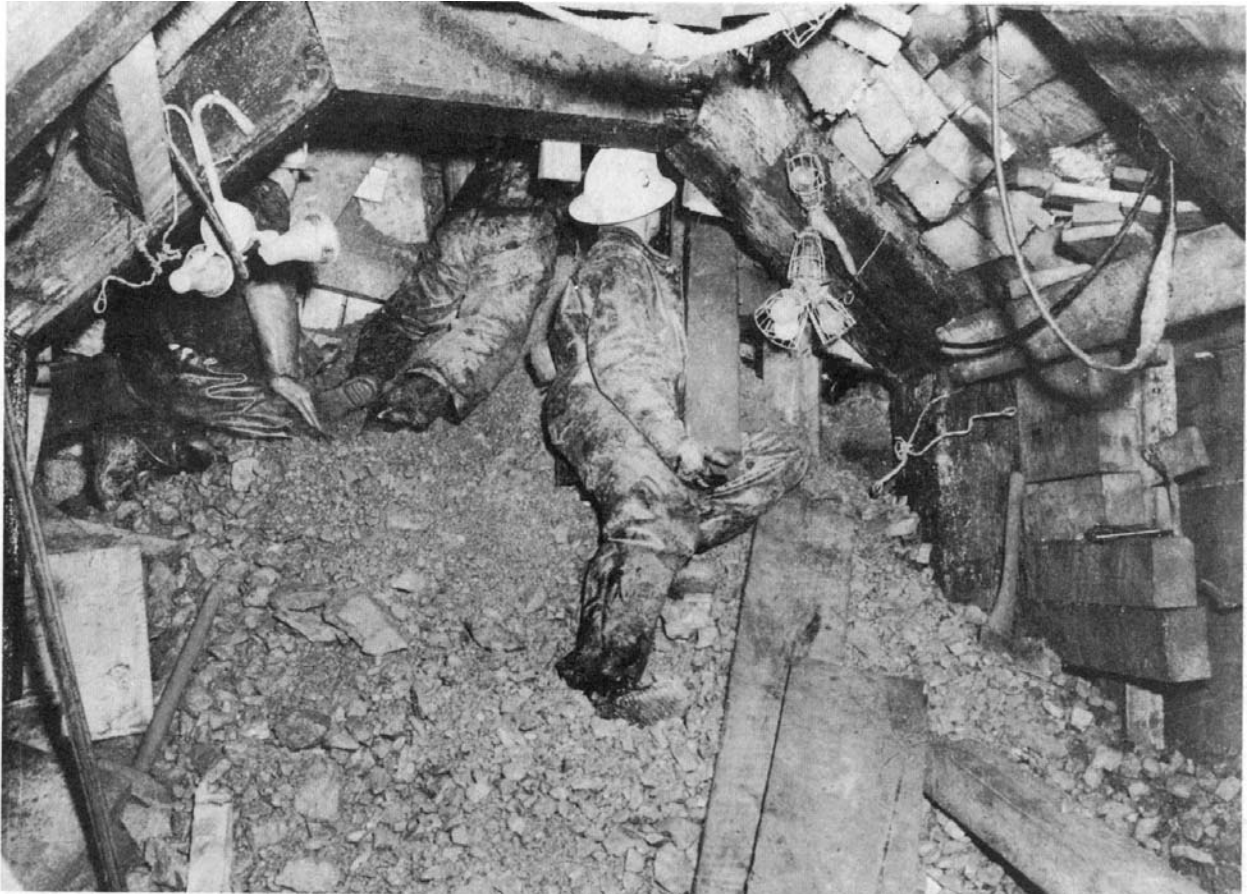
Figure 2. Excavating to remove a boulder at the top of a collapse zone of shattered quartzite in the LMDT, note the mix of material sizes, taken from (Salsbury, 1956).
