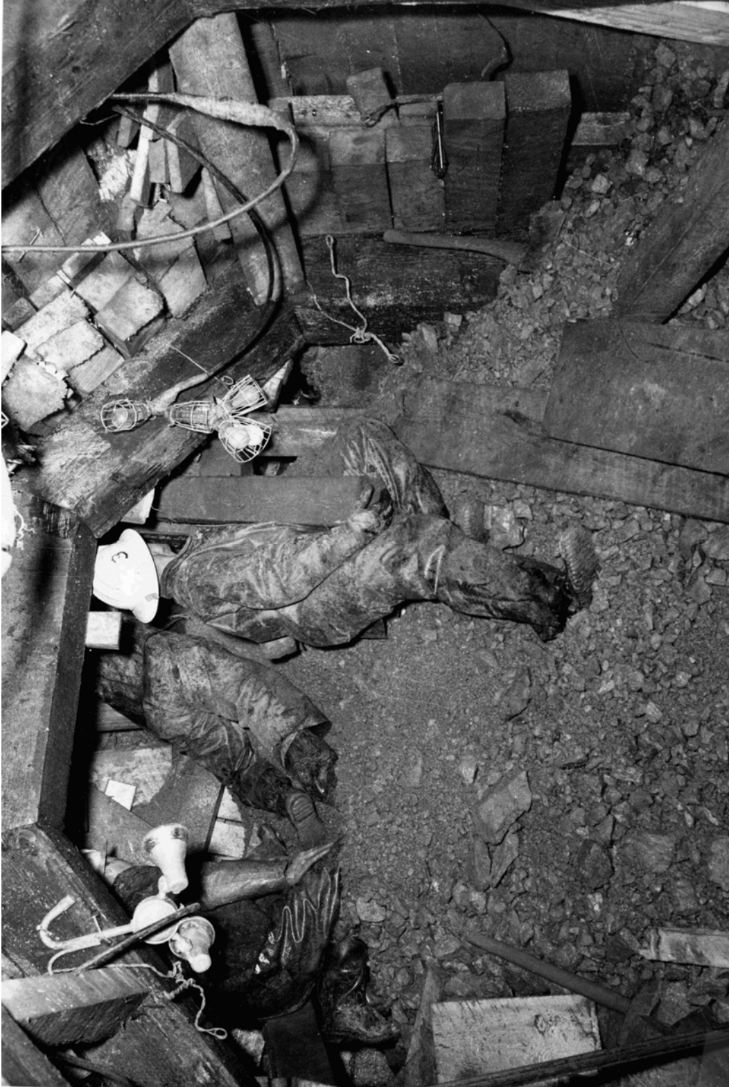
Figure 13. Workers digging out a boulder embedded in running ground in sheared quartzite, taken from (Salsbury, 1956). The boulder prevented spiles from being driven.
