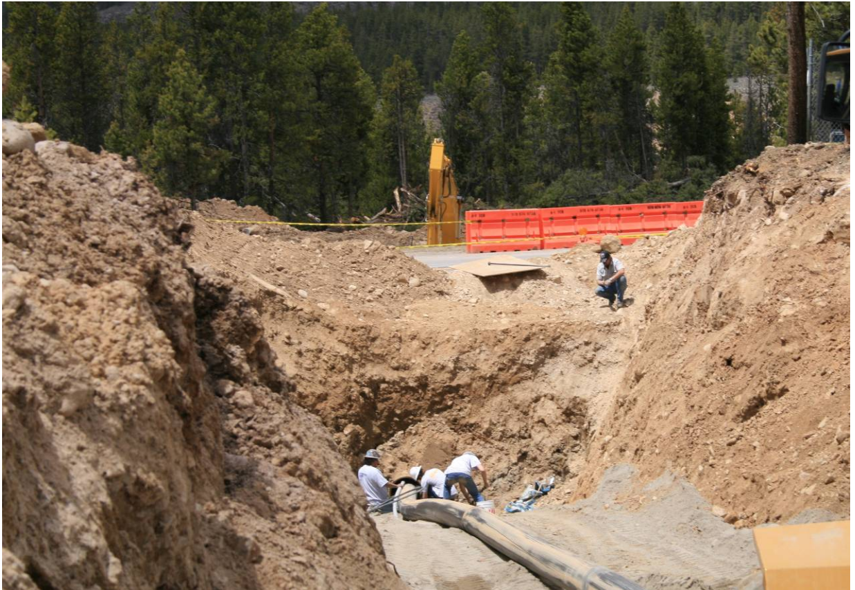
Figure 14. Excavation in May, 2008 into the Glacial Moraine at Leadville for installation of a pipeline under Highway 91 along the alignment of the LMDT. Note the steep slopes of the excavation and spoil banks indicating high shear strength of the soil.
