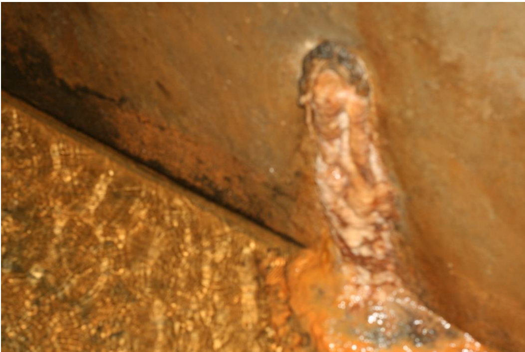
Figure 22. Photograph of a weep hole in the reinforced concrete lining which is almost completely blocked by calcium carbonate precipitates.
