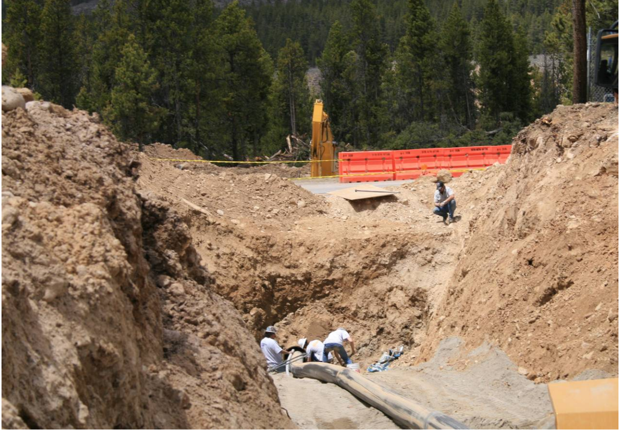
Figure 8. Excavation into the Glacial Moraine at Leadville for installation of a pipeline under Highway 91 along the alignment of the LMDT (late spring 2008)
