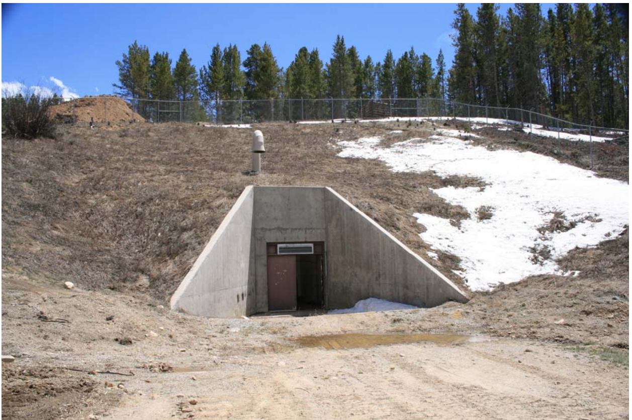
Figure 8. Photograph taken May 21, 2008 showing the reinforced concrete LMDT Portal with 1-ft. thick wing walls.
