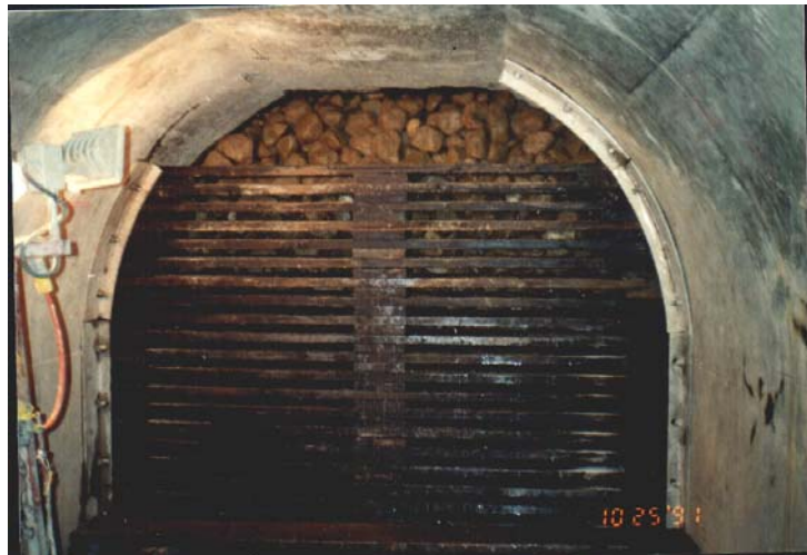
Figure 26. Construction photograph showing the cobbles behind the timber-lattice bulkhead at Station 4+60 of the LMDT.
