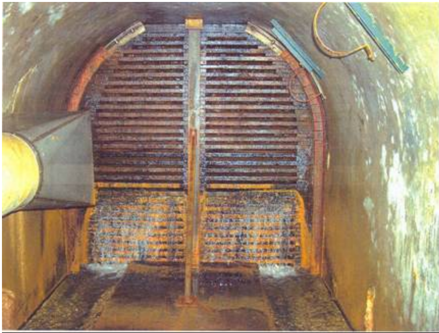
Figure 4. - Photograph taken in 2001 of the existing Timber Lattice Bulkhead installed in 1991 at Station 4+60 to 4+61. Note clarity of water outflow and 2.5-foot high flow with has been typical since post construction.
