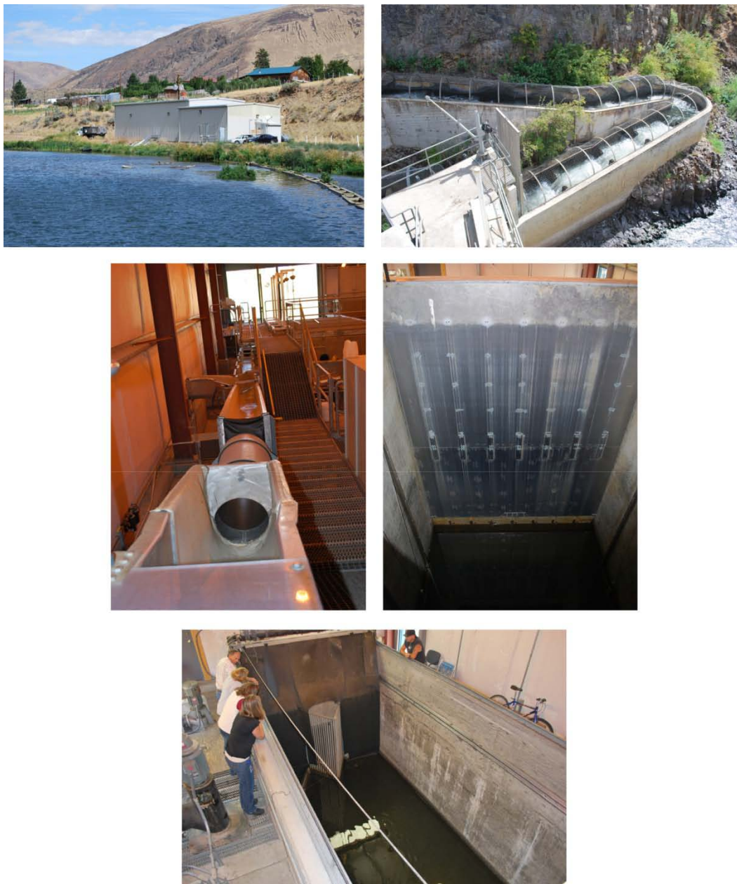
Figure 4-5. View of exterior of Roza adult fish collection facility (top left); pool and weir-type fish ladder (top right); fish chute to work area or back to river (middle left); fish lock (middle right); and adult holding tank (bottom, right)
