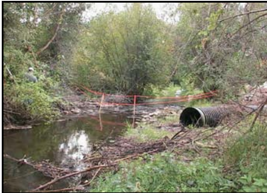
Photo A-4. Looking downstream at entrance to dewatering pipe and the Weir No. 1 layout. The cofferdam will be located between the pipe and the layout.
