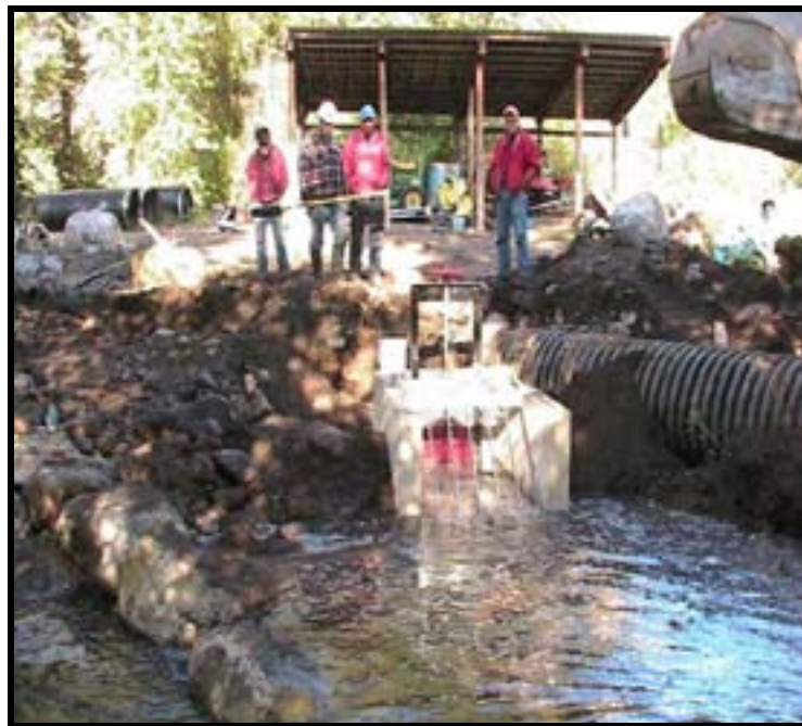
Photo A-14. The newly installed diversion box was tested and satisfied the flow requirement for the landowner's water right.
