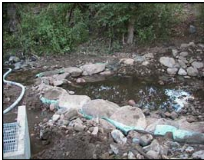
Photo A-12. Completed Weir No. 1. The new diversion box (at lower left) was placed so that it will draw water at low flows but not block water from the right-side weir arm area (foreground).
