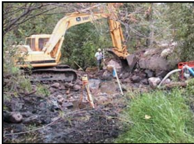
Photo A-20. Looking downstream at initial excavation of Weir No. 3. The concrete at right of photo is the upstream wall of the former diversion dam. The wall and the dam were about the same height (as shown in Photo A-1).
