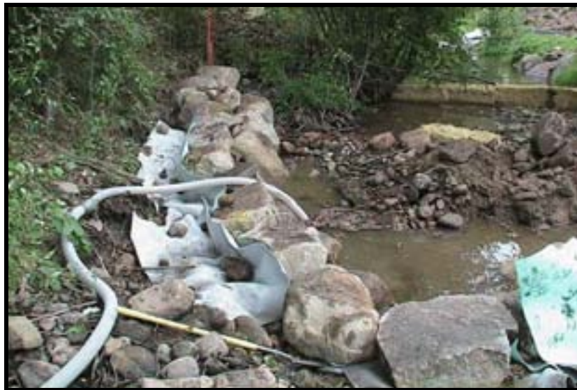
Photo A-8. Installation of geotextile fabric behind first arm of Weir No. 1. Attached to the hose is a trash pump, sending the muddy water up onto the shore so the silt can settle out while the water returns. Note the downstream straw bales.
