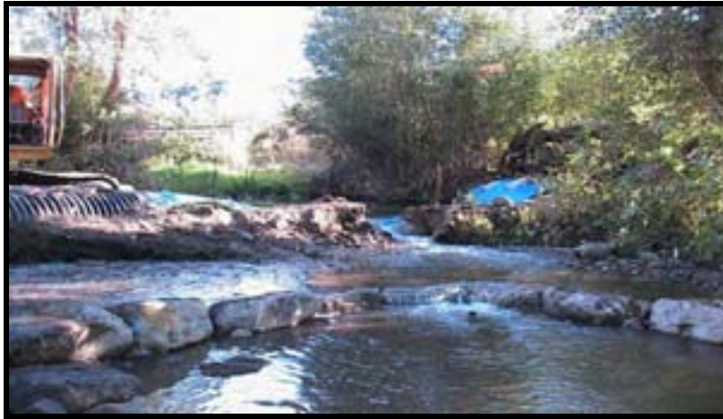
Photo A-13. Looking upstream at newly completed Weir No. 1 and the partially breached cofferdam A. To avoid releasing the backed-up water all at once, the cofferdam is breached in small sections.
