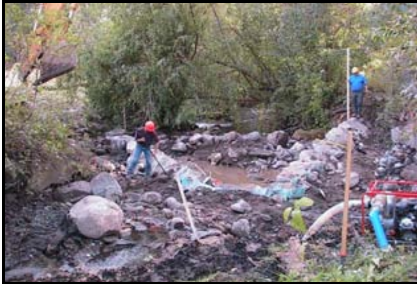
Photo A-21. Looking downstream at Weir No. 3 just prior to completion. The worker at center-left is filling the spaces between the large rocks with cobble-size material and fines.
