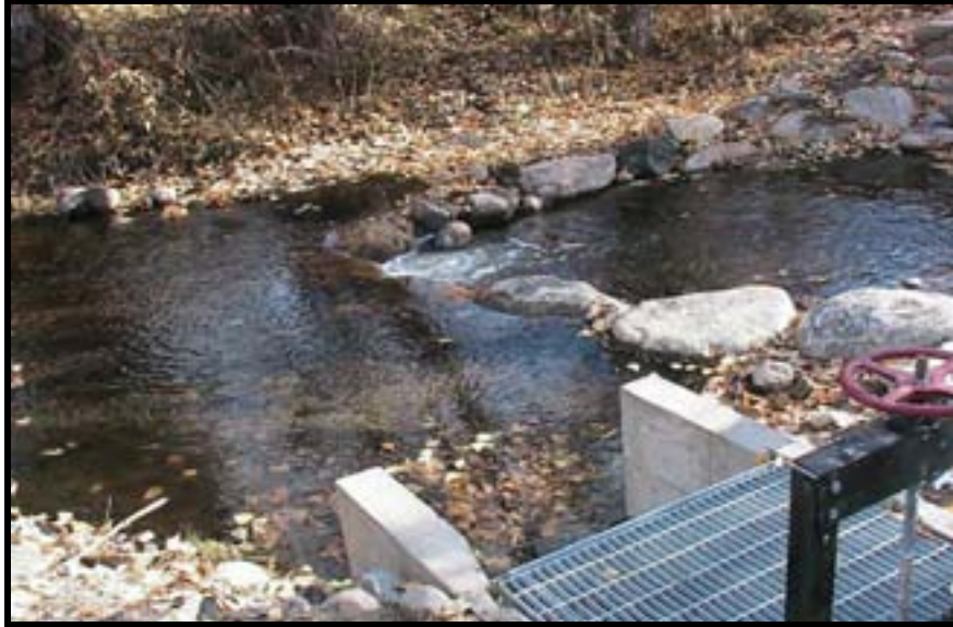
Photo A-25. This picture of Weir No. 1 was taken about mid-November 2003, about 2 months after completion. The weir was designed to pass a “bankfull” flow of 170 cfs and was tested with one minor event of about 30 cfs. The flow shown is about 6 cfs.
