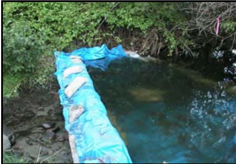
Photo A-18. Cofferdam B with sandbags holding down geotextile tarp, which holds back water.
