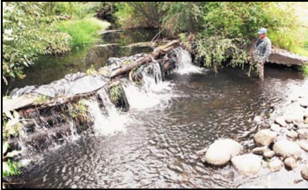
Photo A-1. Original Lower Stokes Diversion Dam just prior to removal; the dam height is about 3½ feet. Compare the concrete wing wall behind worker and the water elevations to that shown in Photo A-20.
