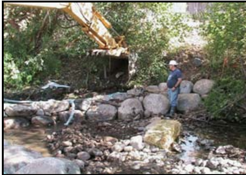
Photo A-10. Backfilling the left-bank weir arm. Note the even slope of the weir arm toward the center of the structure and the lack of spaces between rocks.
