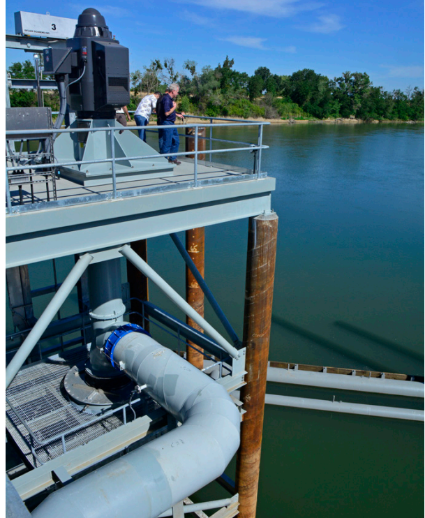
Pritchard Lake Fish Screen and Intake Facility
