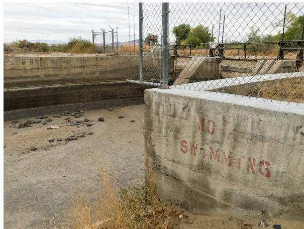
The Lahontan Basin Area Office's empty V-Line Canal headworks on the south side of the Carson Diversion Dam. The 2015 water year saw a 21 percent allocation for the Newlands Project, the lowest recorded allocation in the 110-year history of the project.
