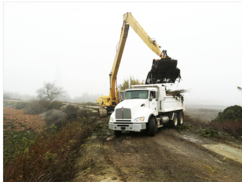
Spoil area re-graded to improve drainage and safety; removed 112,000 cubic yards of hyacinth.
