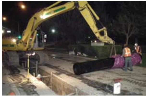
Workers use an excavator to install a recycled-water distribution pipe below a road at night to reduce effects on traffic.
