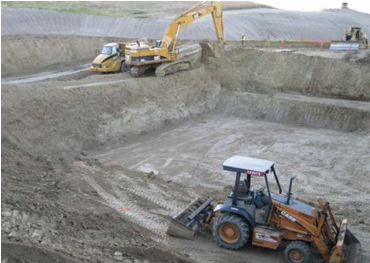
This January 2011 photograph shows excavation work for a pump plant intake for the project.
