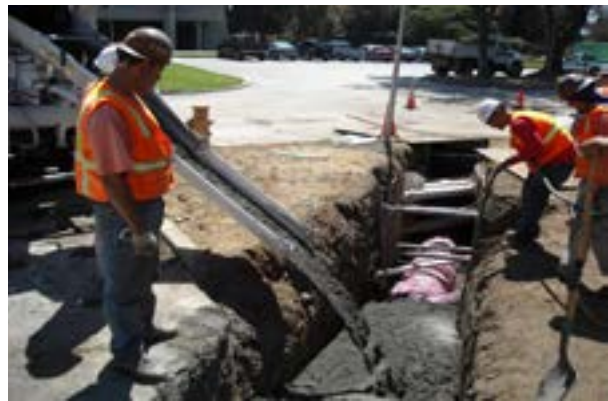
Workers pour concrete over a recycled-water distribution pipe under a street as part of a Palo Alto city project.
