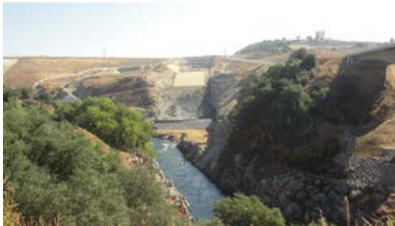
Water released into the new auxiliary spillway, shown at the top, will flow into the American River in the foreground.
