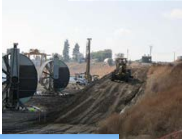
Heavy equipment excavates the canal on the east side of Red Bank Creek.
