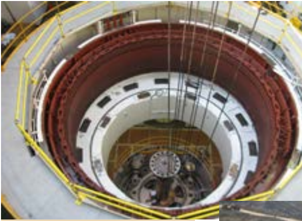
Contractors disassemble part of the equipment related to the hydroelectric power plant at Folsom Dam.
