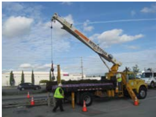
Loads of pipe to convey recycled water are hauled to sites by flat-bed trucks equipped with cranes.
