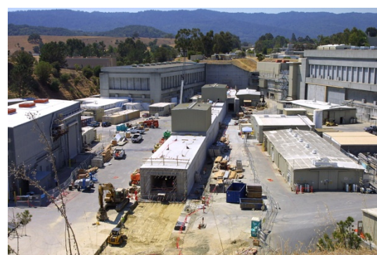
Linac Coherent Light Source (LCLS) Beam Transfer Hall (under construction)
