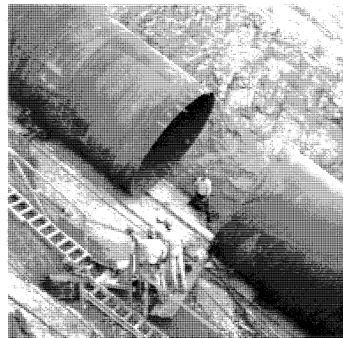
Pipe for the Havasu Pumping Plant discharge line.
