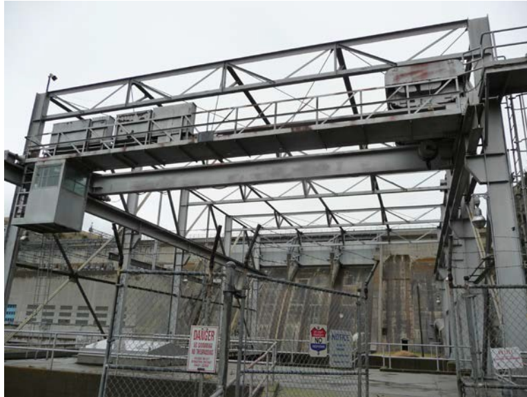
Figure 3. Existing Pumping Plant.
