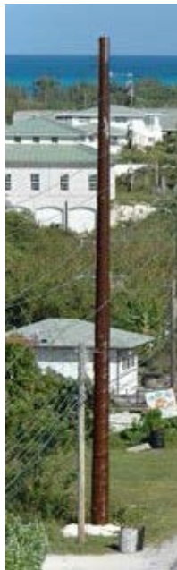
Figure 8. Typical weathered pole.
