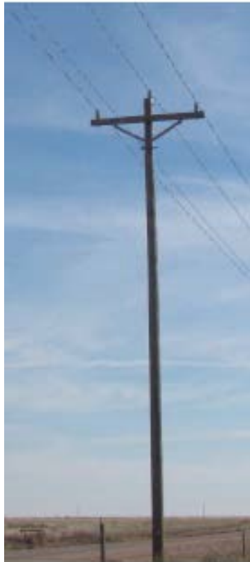
Figure 12. Typical Distribution Line Pole.
