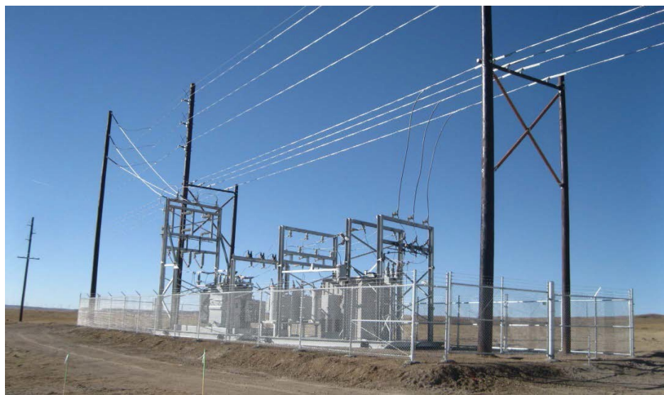
Figure 9. Example of Skid Mounted Substation
