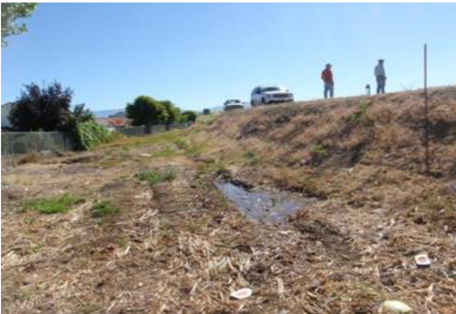
Figure 10. Ponded water and moist soil near toe of the canal embankment.
