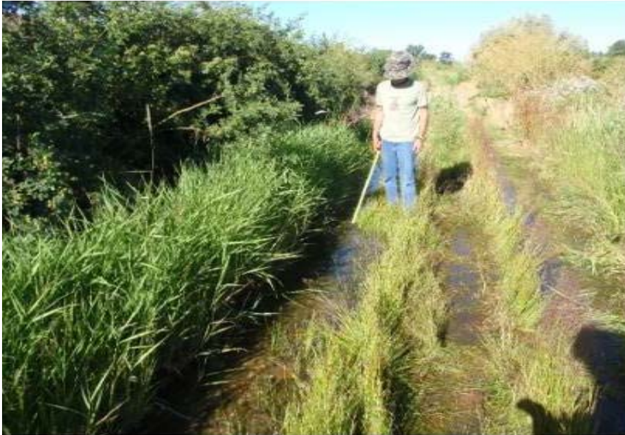
Figure 9. Active seepage area near the outside of the canal embankment.
