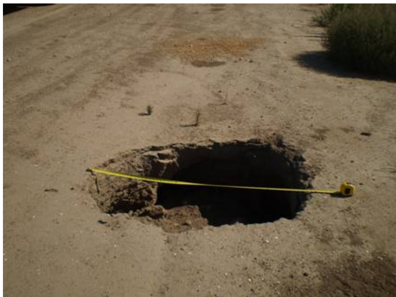
Figure 15. Void on the crest of the canal embankment.
