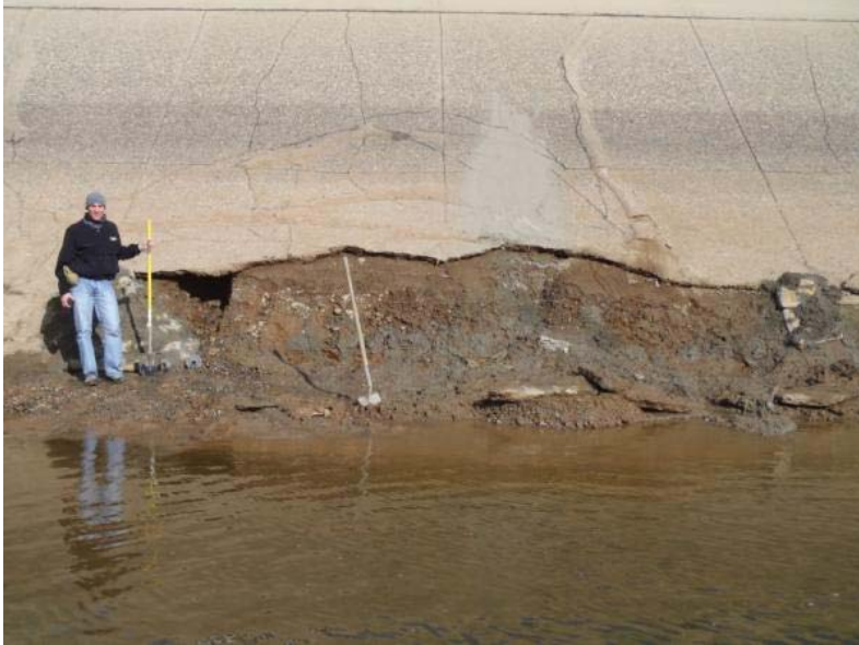
Figure 19. Distressed canal lining on the inside slope of the canal prism observed during dry inspection.
