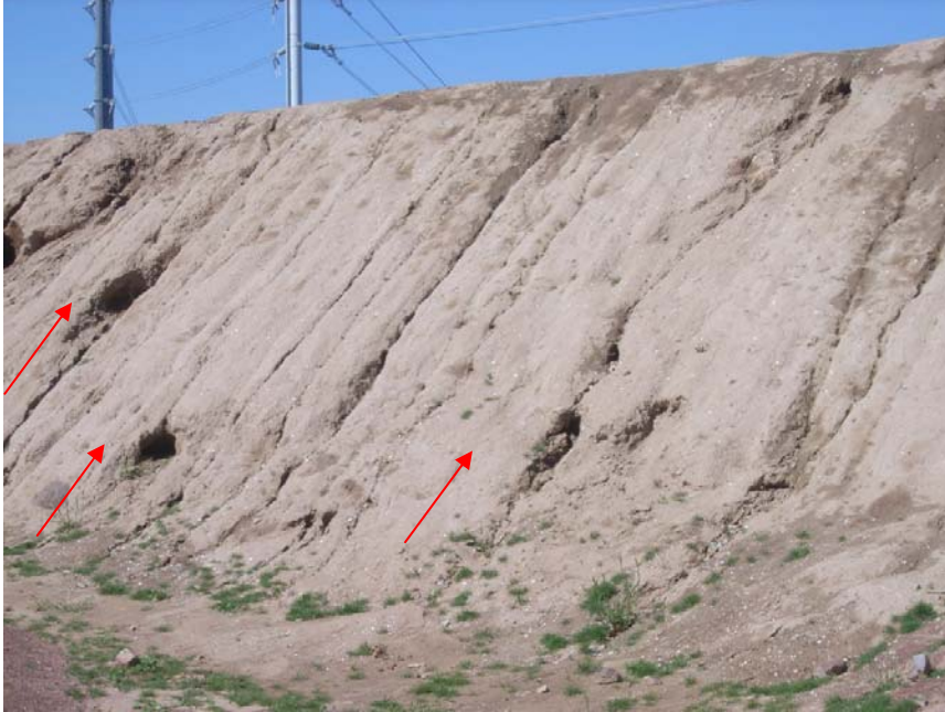
Figure 11. Large and small diameter animal burrows on the outside of the canal embankment.
