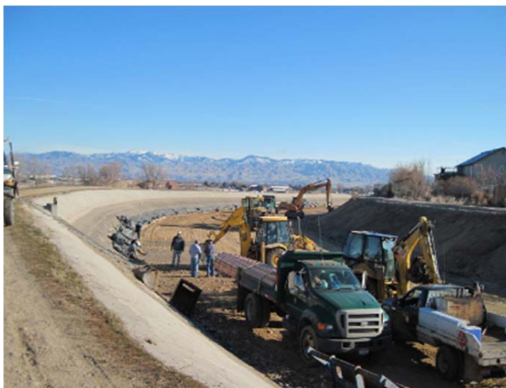
Figure 22. Operating entity performing repairs to address a seepage area.
