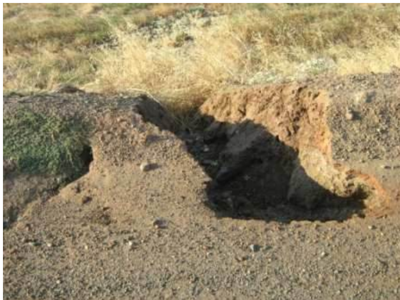
Figure 16. Erosion of outer slope of the canal embankment.
