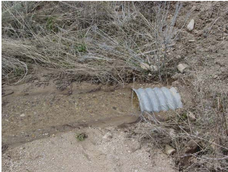
Figure 21. Plugged corrugated metal pipe culvert that is limiting cross drainage.
