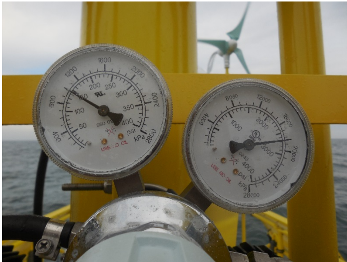
High and low pressure gauges
