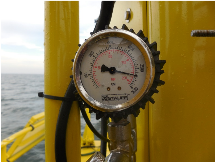
Starboard air tank pressure level
