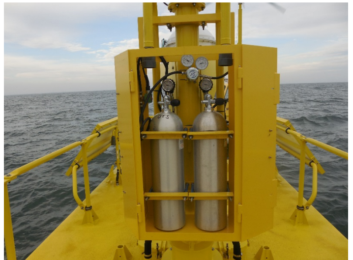
Pressurized air system
