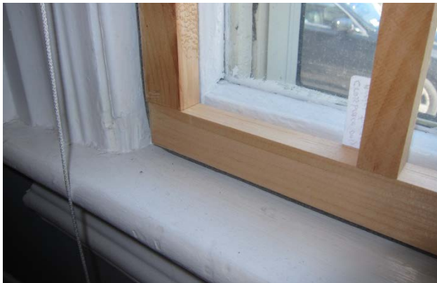
Figure 26. Installed interior removable storm window
