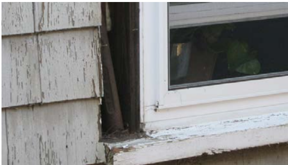
Figure 17. Sash weight pockets
