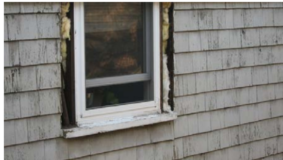
Figure 18. Abandoned sash weight and insulation installation
