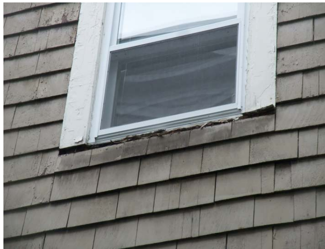
Figure 5. Failed window sill with replacement window installed
