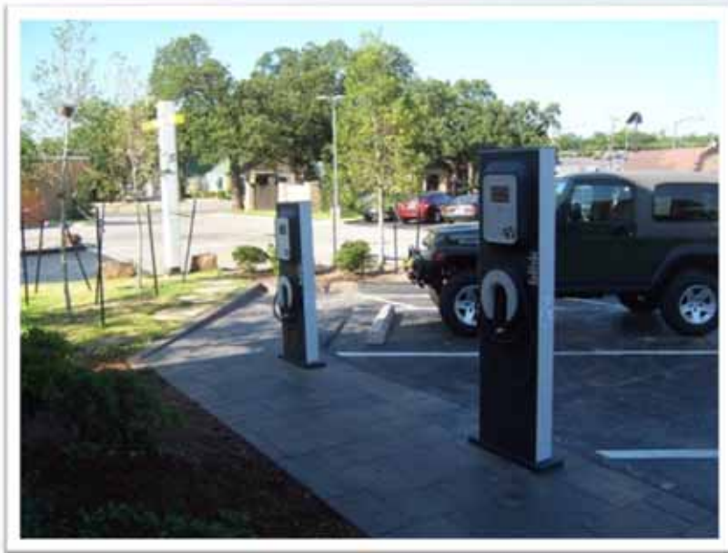
Pedestal EVSE installed on decorative paving; removal and replacement required for underground conduit
