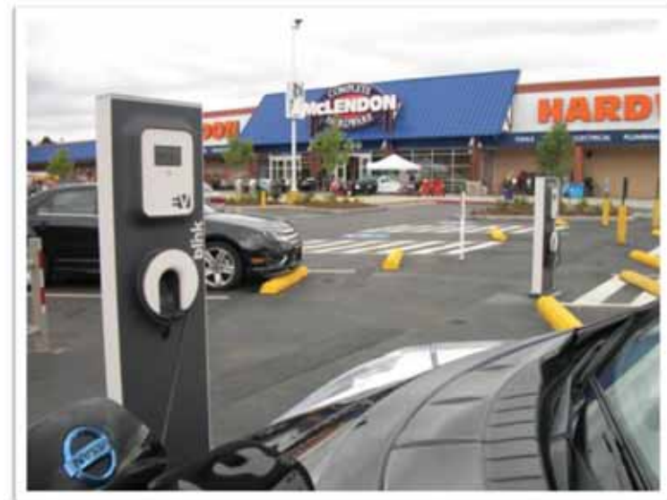
Pedestal EVSE installed on asphalt, with trenching and repaving for underground conduit
