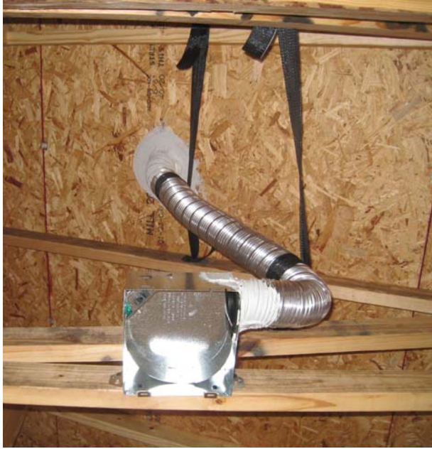
Figure 3. Duct sealing and smooth bends make for a good local exhaust installation
