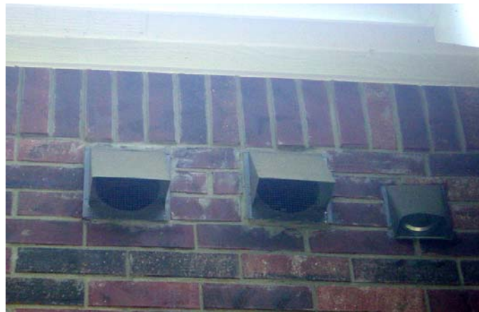
Figure 6. Keep exhaust outlets (small wall cap shown on right) at least ten feet away from outside air inlets (larger wall caps shown on left)
