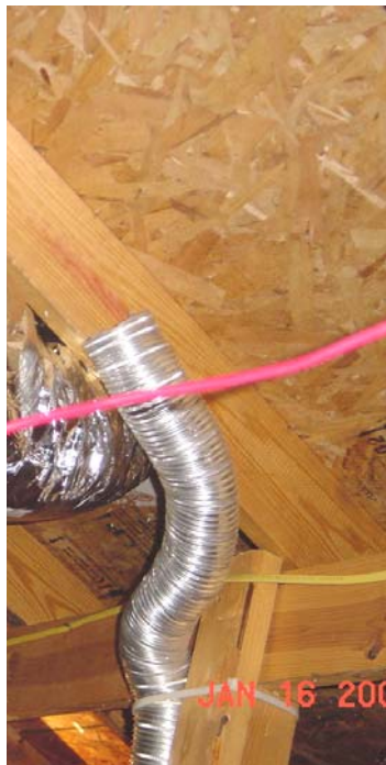
Figure 2. Terminating a local exhaust duct in the attic is not acceptable
