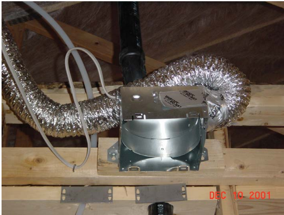
Figure 4. Sharp duct bends dramatically reduce airflow, and cloth-backed duct tape does not hold for the long-term
