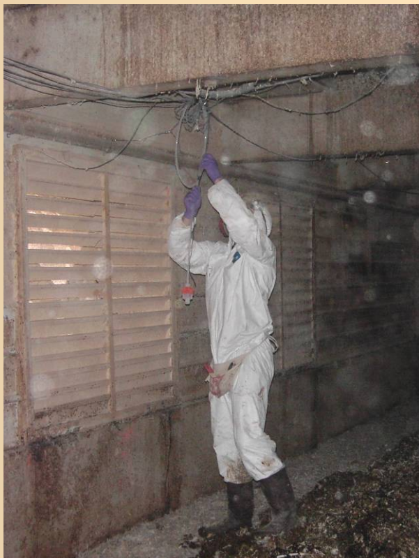
Installing sampling line and port at a fan in the lower level of the HR barn
