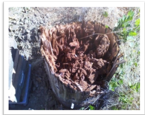
Figure 1-2. Decayed Wood Pole
