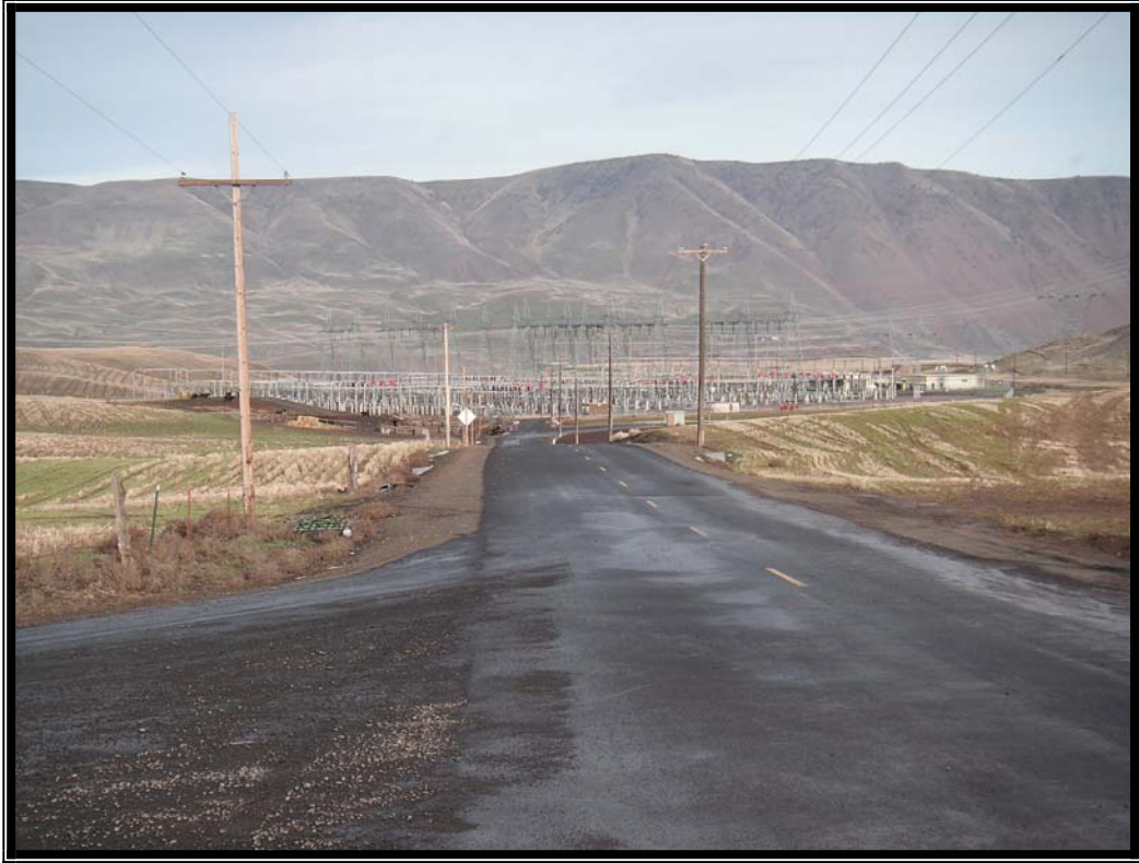
PHOTO 1: John Day Substation looking north.
