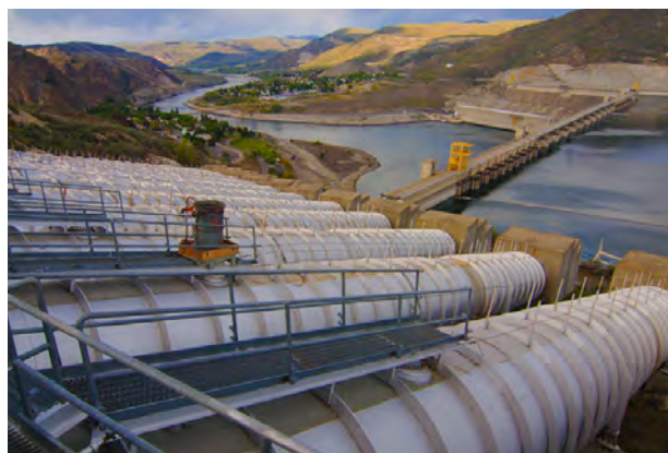
Figure 11: Photo of Grand Coulee John W. Keys III Pump-Generating Plant.
