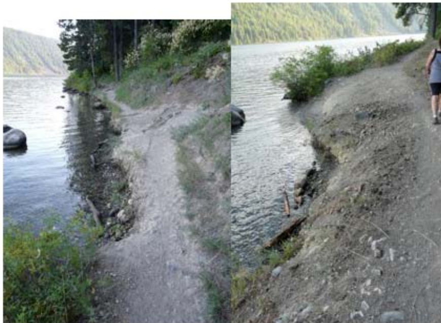
Shoreline Trail This is typical of the extreme erosion that occurs all along the trail.
