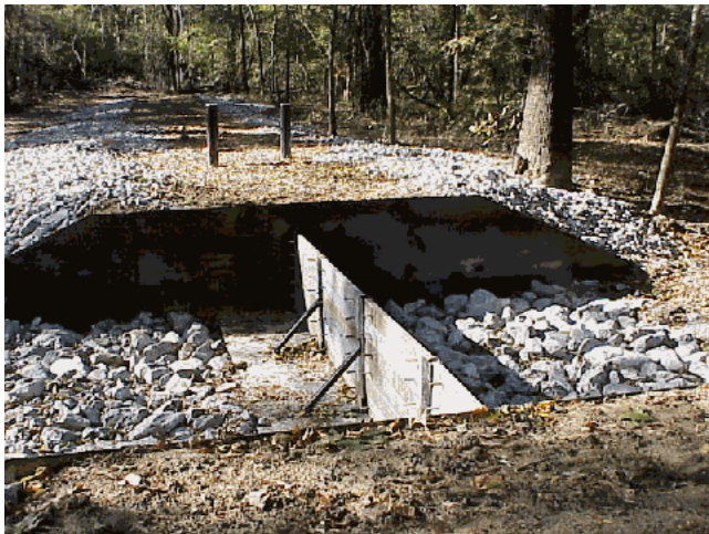
Figure I.C.1-3 Open flow straight drops (photo courtesy of Bobby Massey, Ducks Unlimited)
