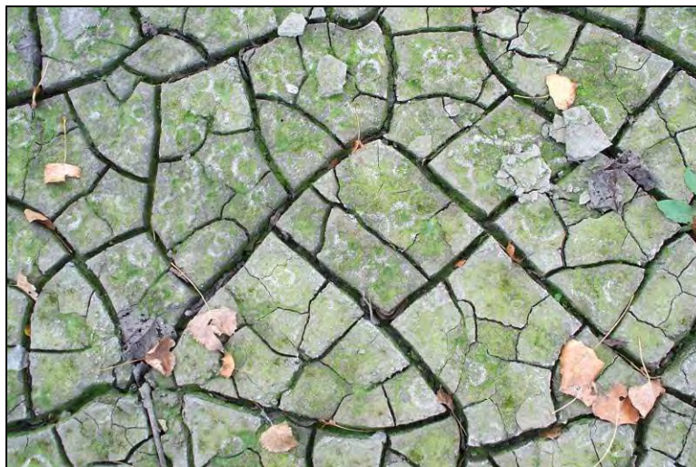
Figure 50. Surface soil cracks in a seasonally ponded depression.
