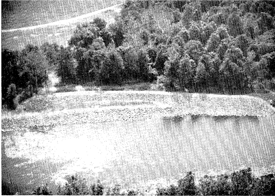
FIGURE 12. ROCK RIPRAP SPUR; LOYALSOCK CREEK NEAR MONTOURSVILLE, PA. (COURTESY, PENNSYLVANIA DEPT. OF TRANSPORTATION, DISTRICT 3-0)
