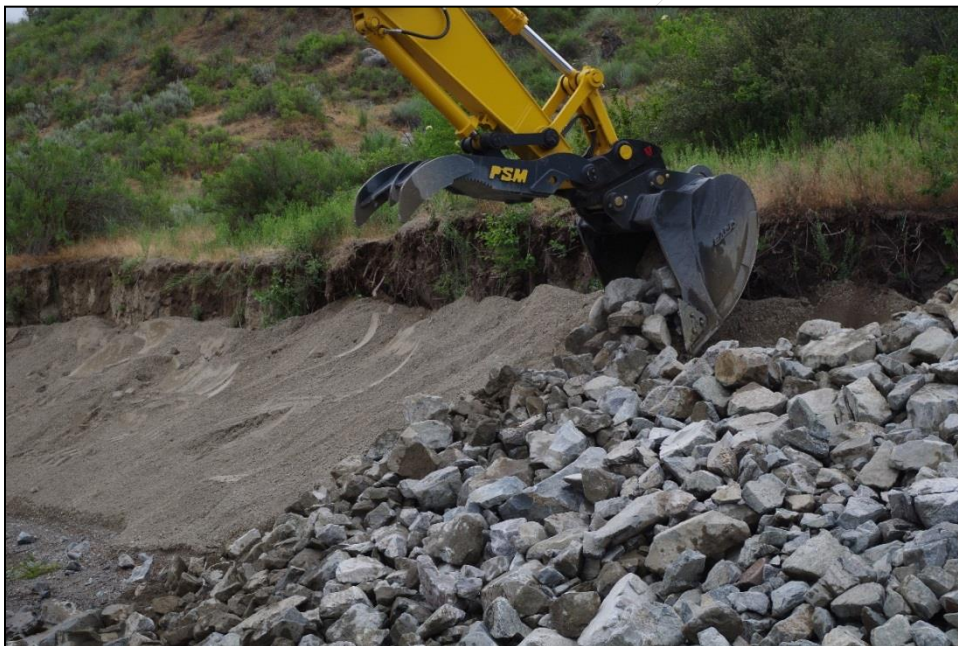
Figure 16. Placing riprap, the next layer, west end of 45-OK-196/197; view to northwest.
