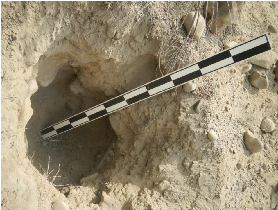
Figure 18. Site Utility Upgrade Corridor Geological Test Hole CJD-15-BH-03, showing deep fill in the Project administrative area.
