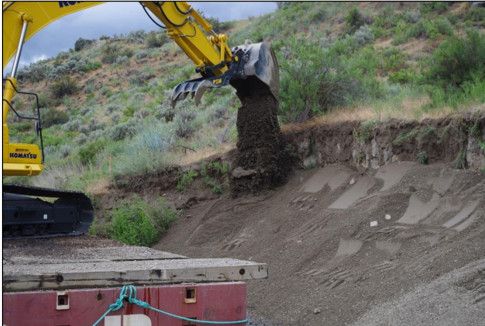
Figure 15. Placing the initial layer of the erosion control structure at the west end of 45-OK-196/197; gravel pad to fill voids and support placement of the riprap. View to northwest.
