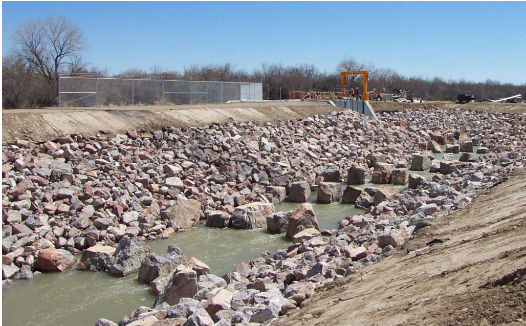
Figure 5—Public Service Company of New Mexico Diversion Dam Rock Fish Passage on the San Juan River, New Mexico
