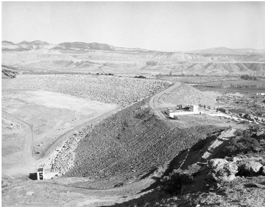
Figure 0.6 Nearly completed dam. View towards right abutment. Project photograph P325-418-0398, photograph by Elmer S. Davis, 10/26/1960.
