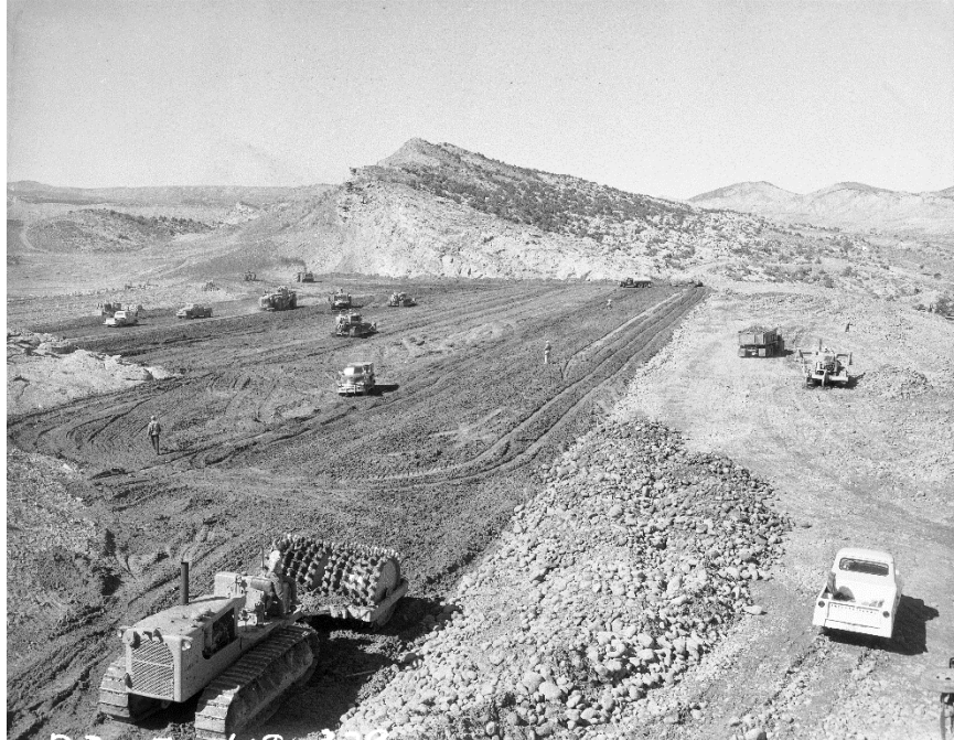
Figure 0.5 Embankment construction in progress on Zones 1, 2, and 3. View is looking northeast from right abutment. Average elevation for the three zones shown is 5450. Project photograph P325-418-0329, photograph by Elmer S. Davis, 7/18/1960.
