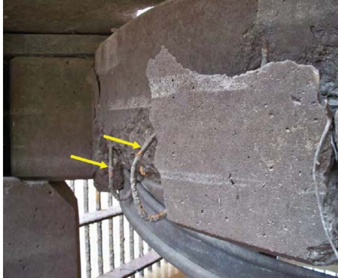
Figure 3. Photograph of some of the damage to the Paonia Dam intake structure bulkhead. Yellow arrows show exposed rebar.
