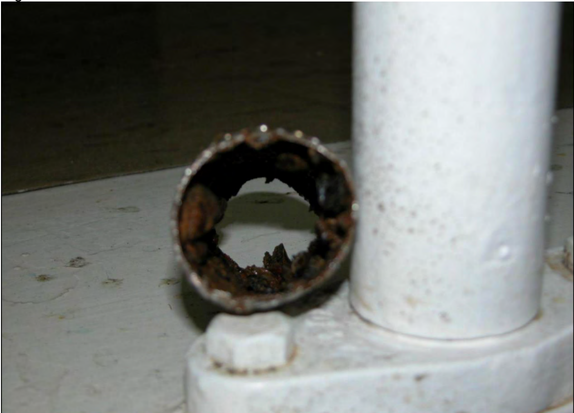
Figure 7. Unit 1 turbine bearing oil heat exchanger Y strainer.
