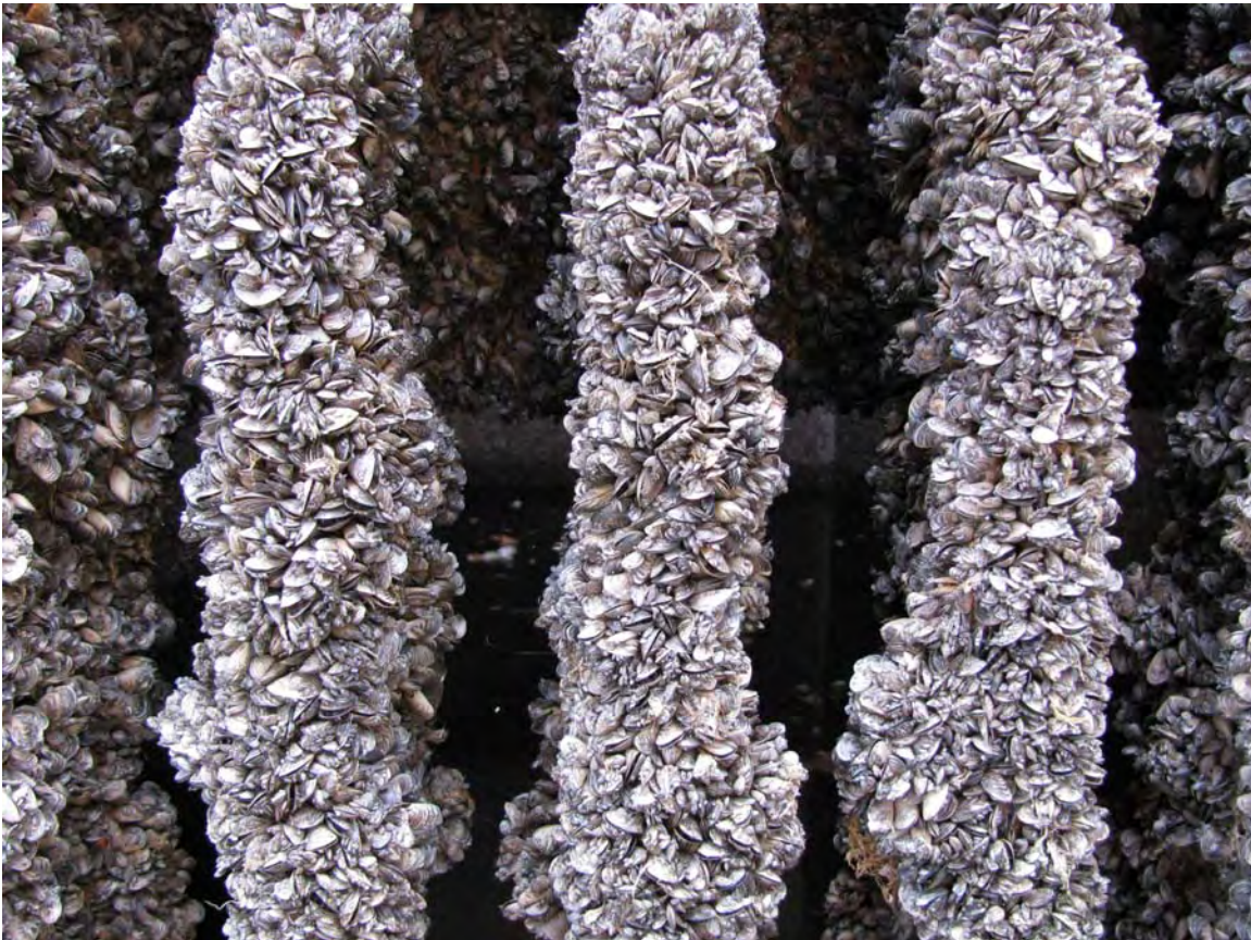
Figure 2. Quagga mussels on intake trashracks at Hoover Dam.
