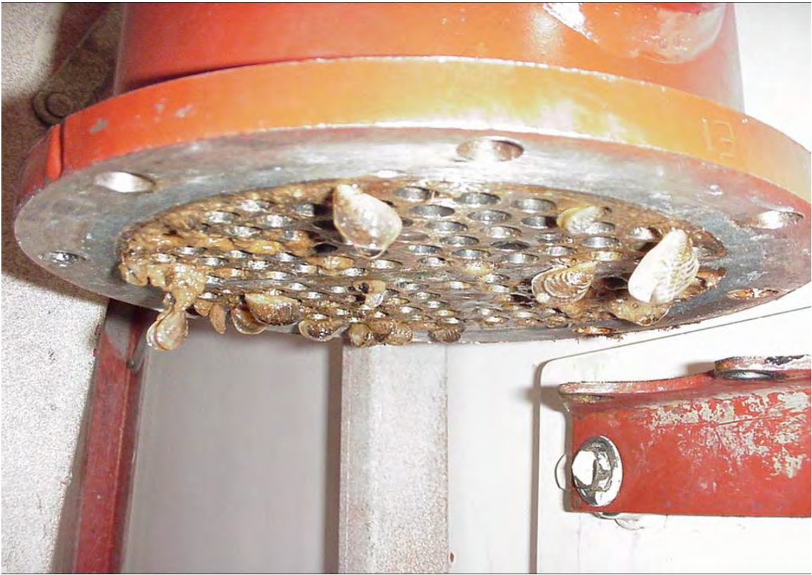
Figure 8. Unit 1 turbine bearing oil heat exchanger, holes are 7/16".
