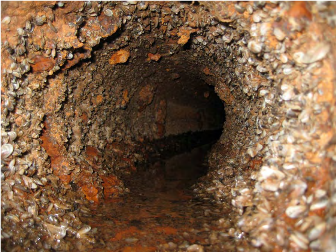
Figure 12. 8" cooling water supply line on Hoover Dam Generator (Nevada #8), November 2008.
