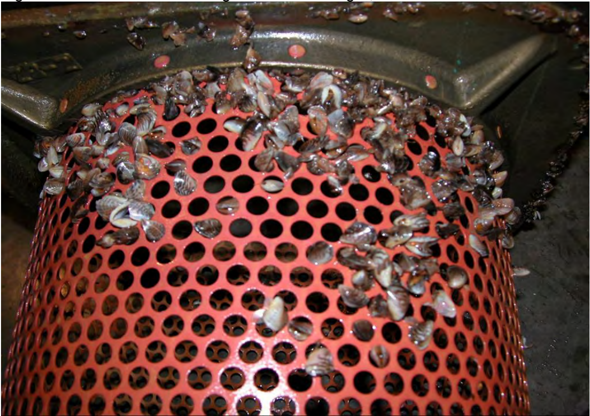
Figure 9. Old style strainer basket pulled from service for inspection.
