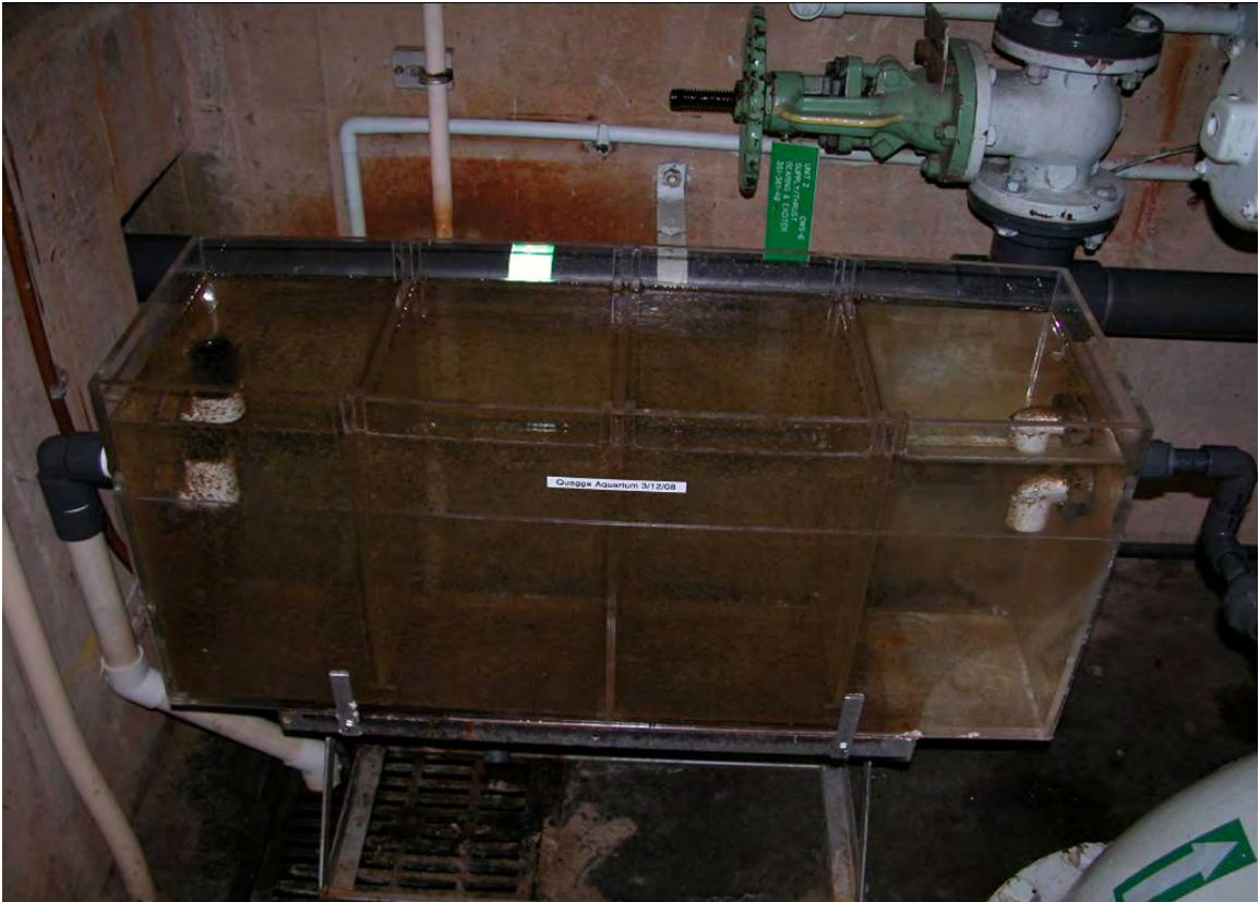
Figure 11. Unit 2 cooling water intake, quagga monitoring tank, 6/26/08
