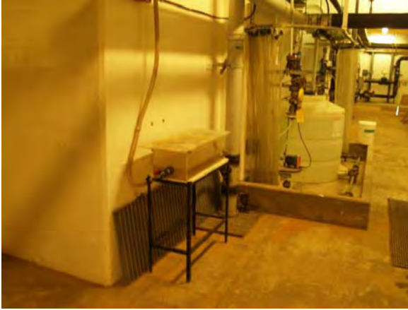
Figure 4: Existing Holding Tank & Injection System, Control Biobox in Foreground
