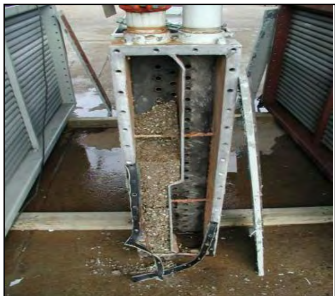
Figure 4. Dead invasive mussel debris in a cooling unit in Ontario, Canada similar to the cooling water system at Davis Dam.
