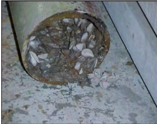
Figure 6. Pipe clogged with quagga mussels in a similar unit in Ontario, Canada.
