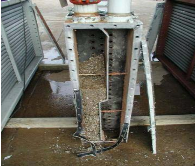
Figure 3. Dead invasive mussel debris in a cooling unit in Ontario, Canada similar to the cooling water system at Davis Dam.
