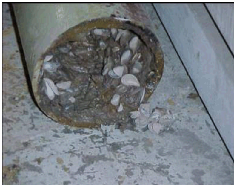
Figure 2. Pipe clogged with quagga mussels in a similar unit in Ontario, Canada.
